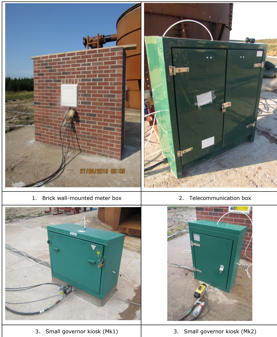
Figure 1: Example Meter Installations and Kiosks tested in H21 Phase1b
