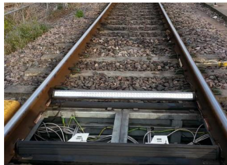
In use within Chiltern Railways depot.
