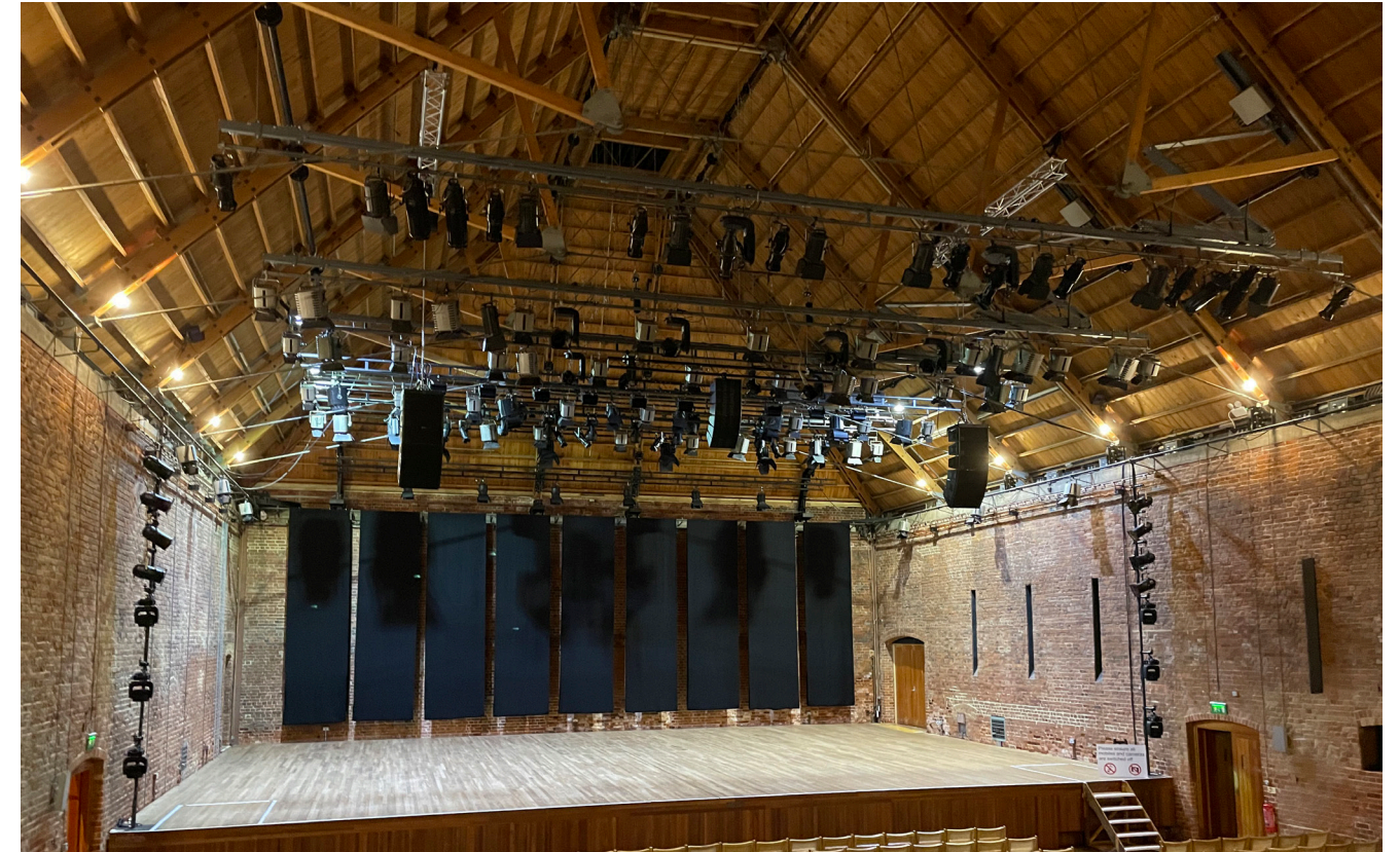
Existing lighting rig within Concert Hall
