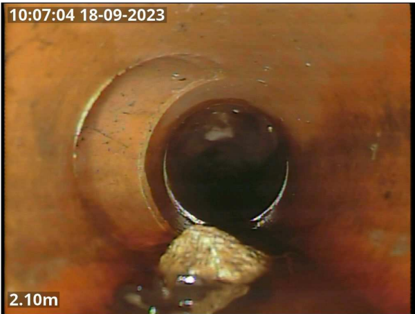
Photo: CCTV 08 pic 1.jpg 2.1m, Junction, at 9 o'clock, diameter 100mm
