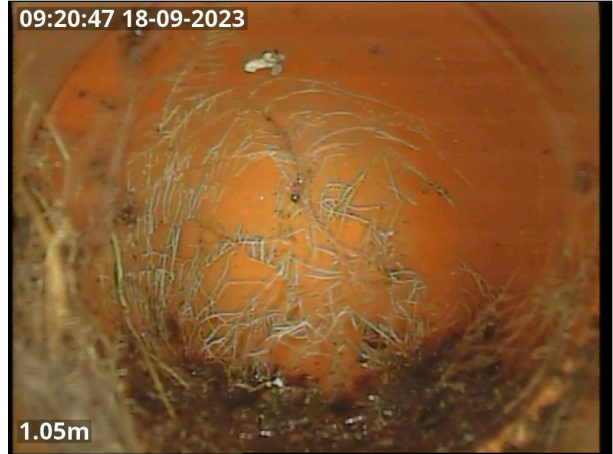
Photo: CCTV 03 pic 2.jpg 1.05m, Finish node type, manhole reference number: Lateral 1
