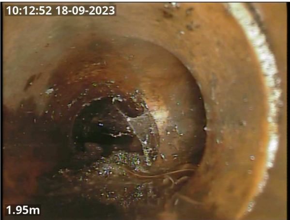
Photo: CCTV 09 pic 1.jpg 1.95m, Junction, at 2 o'clock, diameter 100mm
