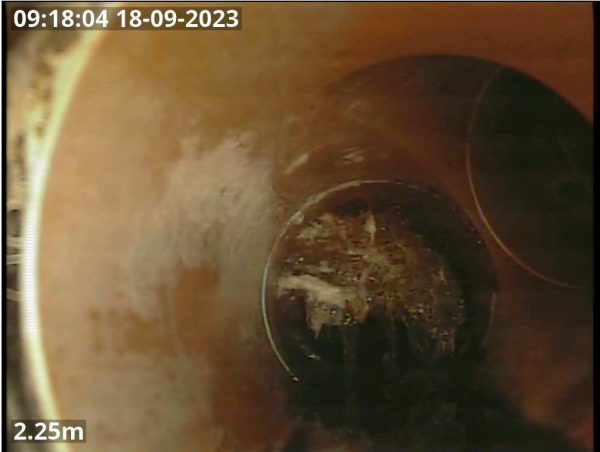
Photo: CCTV 02 pic 1.jpg 2.25m, Junction, at 2 o'clock, diameter 100mm
