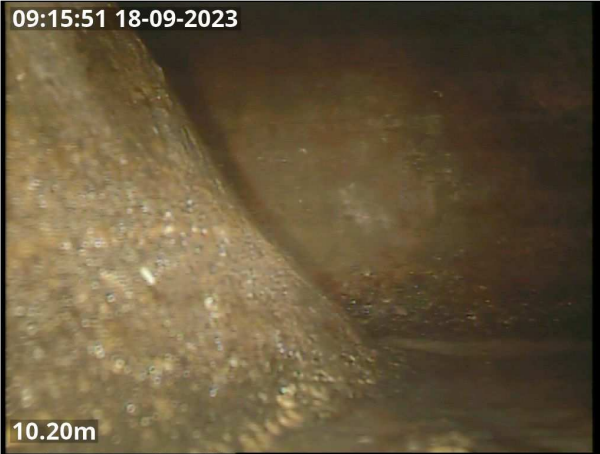
Photo: CCTV 01 pic 1.jpg 10.2m, Finish node type, manhole reference number: MH 3
