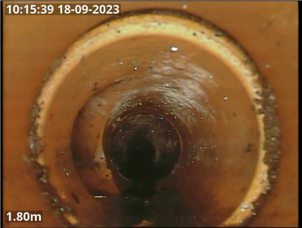
Photo: CCTV 10 pic 1.jpg 1.8m, Junction, at 3 o'clock, diameter 100mm
