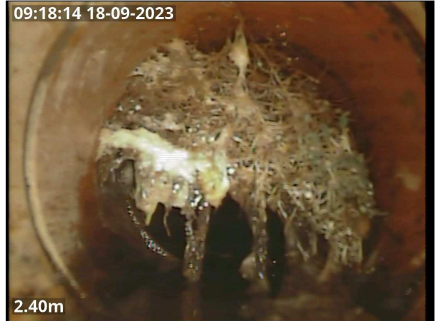
Photo: CCTV 02 pic 2.jpg 2.4m, Survey abandoned
