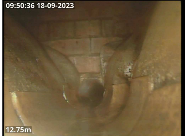
Photo: CCTV 05 pic 2.jpg 12.75m, Finish node type, manhole reference number: MH 5
