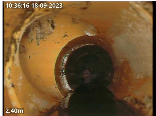
Photo: CCTV 12 pic 2.jpg 2.4m, Junction, at 9 o'clock, diameter 100mm
