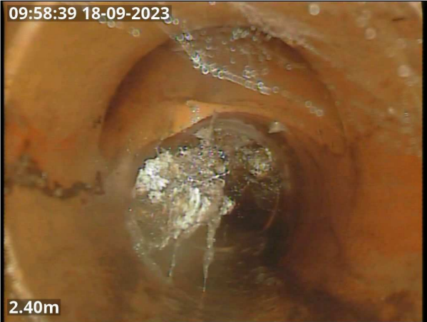
Photo: CCTV 07 pic 1.jpg 2.4m, Junction, at 12 o'clock, diameter 100mm
