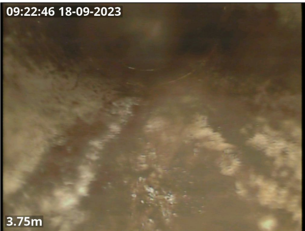
Photo: CCTV 04 pic 3.jpg 3.75m, Finish node type, manhole reference number: Lateral 2
