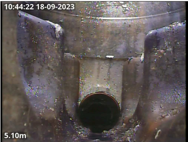
Photo: CCTV 13 pic 1.jpg 5.1m, Finish node type, manhole reference number: MH 2
