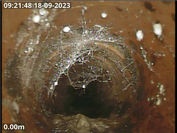
Photo: CCTV 04 pic 1.jpg 0m, Settled deposits, fine, 5% cross-sectional area loss
