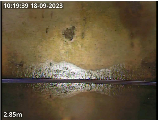
Photo: CCTV 11 pic 1.jpg 2.85m, Finish node type, manhole reference number: Lateral 2
