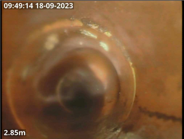
Photo: CCTV 05 pic 1.jpg 2.85m, Junction, at 2 o'clock, diameter 100mm
