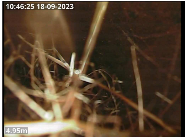
Photo: CCTV 14 pic 2.jpg 4.95m, Finish node type, manhole reference number: Upstream
