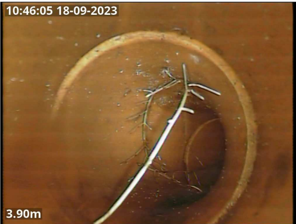
Photo: CCTV 14 pic 1.jpg 3.9m, Roots, fine
