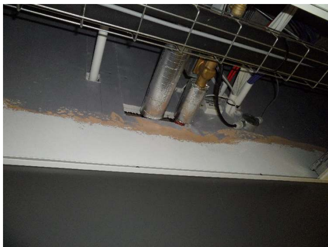
19. Un-stopped service penetrations
