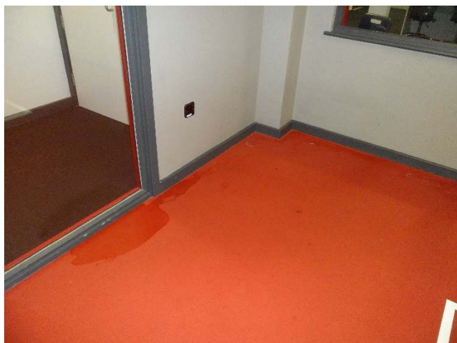
27. Staining to gym floor
