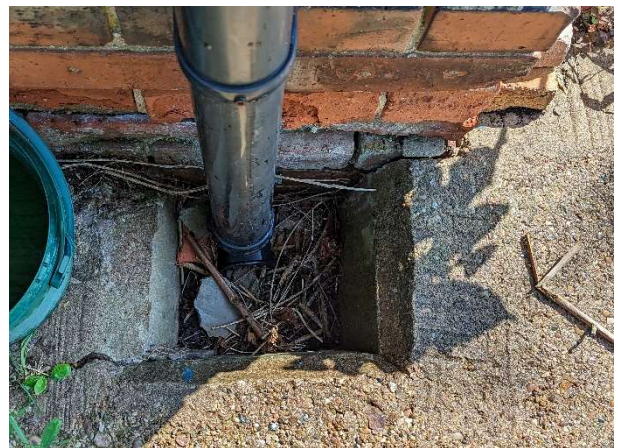
Photo 10 – Drainage channel blocked by debris on the western elevation.
