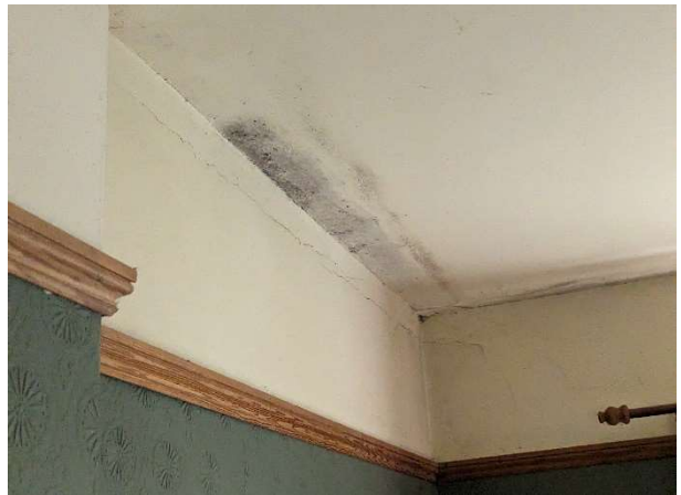
Photo 60 – Black mould present to ceiling and walls.
