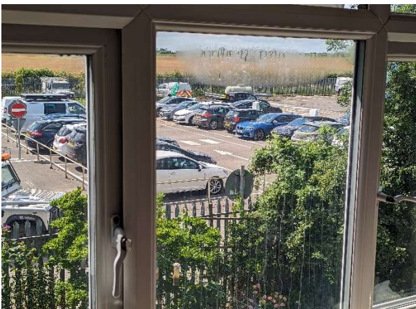
Photo 51 – Blown glazing panel to window unit located in Bedroom 2.
