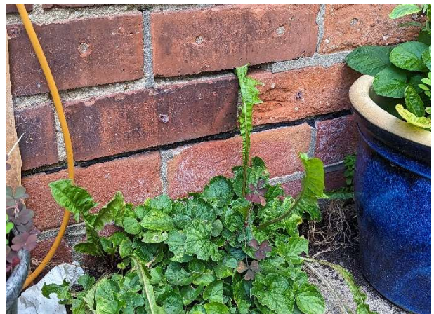
Photo 4 – Missing mortar throughout the exterior of the building.
