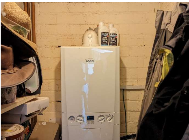
Photo 47 – Boiler located in the Pantry located in the rear porch area.
