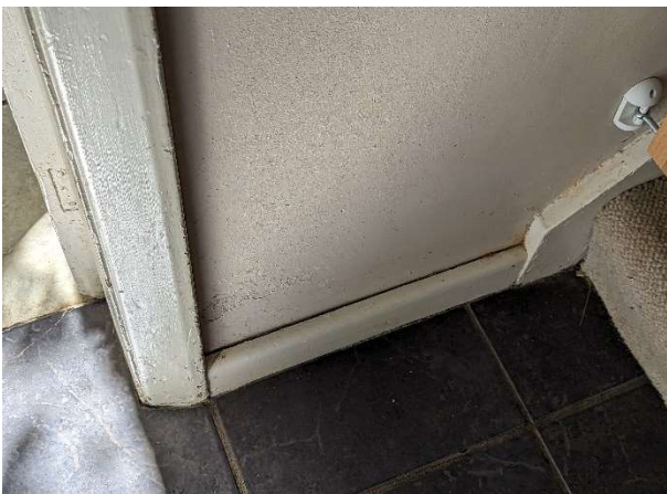
Photo 35 – Blistering and elevated moisture levels to walls at low level of front porch area,
