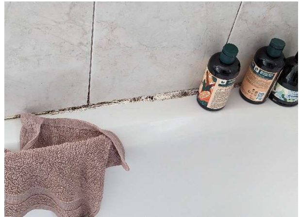
Photo 40 – Mildew build up to grouting around tiles and bathtub.
