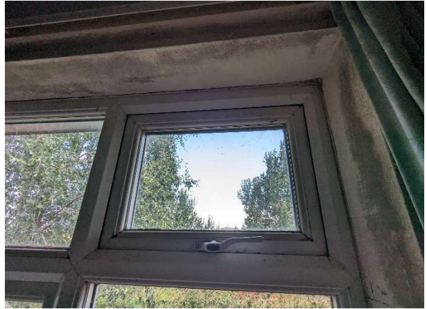
Photo 56 – Black mould to window reveal.
