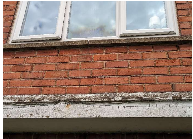
Photo 2 – Horizontal crack at upper level to the front elevation.
