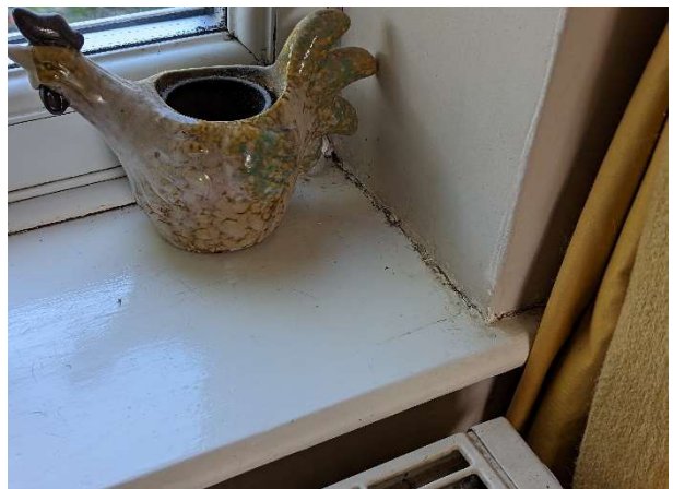
Photo 34 – Closer view of window sill and boards.
