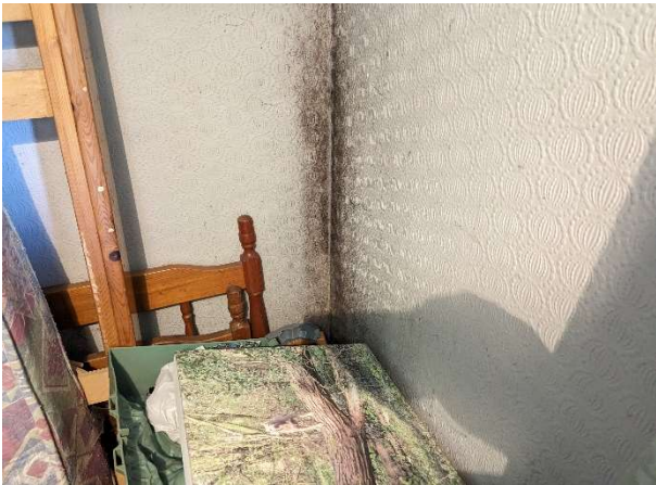
Photo 57 – Black mould to walls and ceilings to Bedroom 3.
