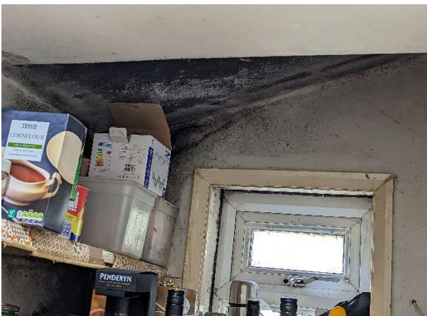
Photo 45 – Black mould to wall/ceiling to the Pantry located in the kitchen.
