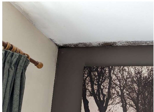
Photo 52 – Black mould to ceiling and walls, predominantly in the corners of Bedroom 2.
