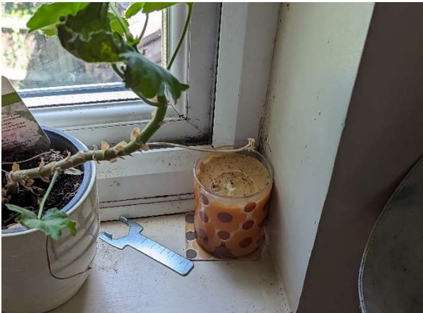
Photo 49 – Close up of black mould affecting the window reveal of Bedroom 2.
