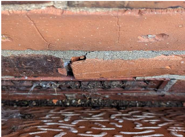
Photo 7 – Example of airbricks blocked by a clay panel.
