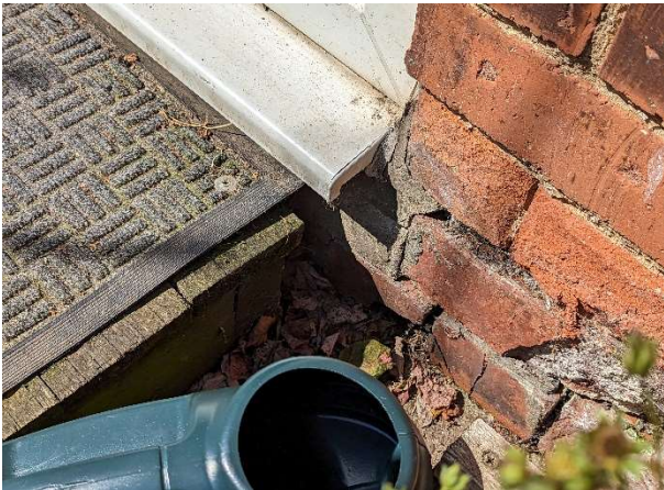
Photo 19 – Further examples of mortar missing at low level.
