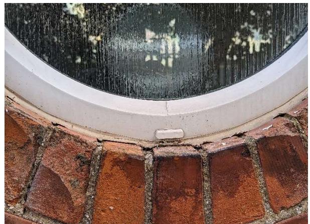
Photo 6 – Mastic/Sealant become loose to several windows.
