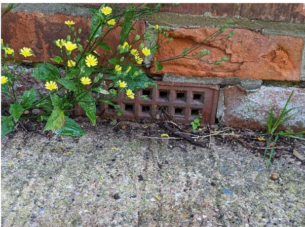
Photo 9 – Airbricks partially blocked by paved concrete on the western elevation.
