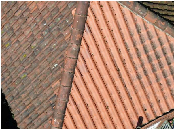
Photo 27 – Closer view of the ridge tiles and condition.
