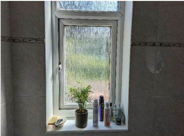
Photo 39 – Blown glazing panel to bathroom window.
