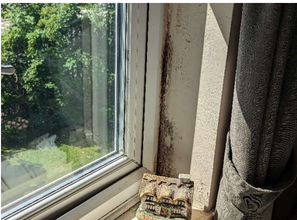
Photo 53 – Black mould to window reveal to Bedroom 2.
