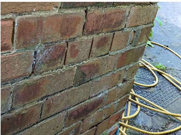
Photo 15 – Further examples of mortar missing at low level.
