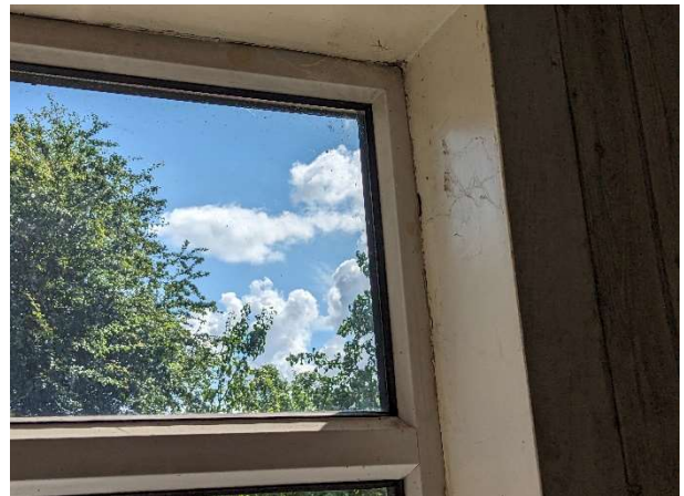
Photo 42 – Flaking paint to window reveal at high level.
