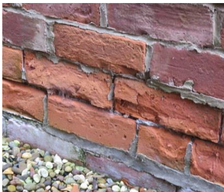
Low level brickwork spalled and pointing poor.
