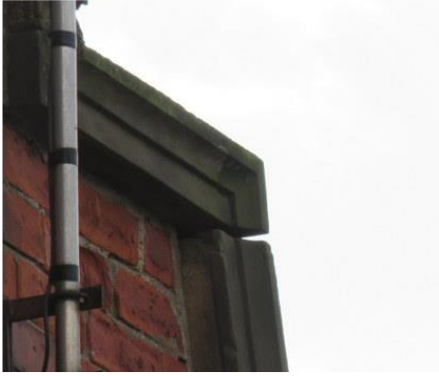
Open joints to gable parapet capping stones.
