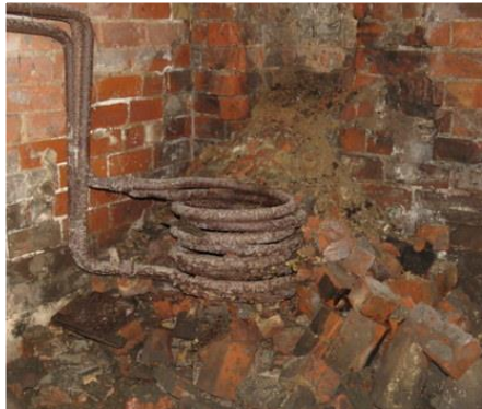
Redundant heating coil to perimeter underfloor heating.
