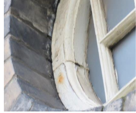
Seal around wooden windows have perished.
