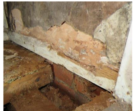
Rot to floor and skirtings in kitchen.
