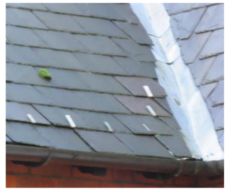
Tingles evident to entrance roof.
