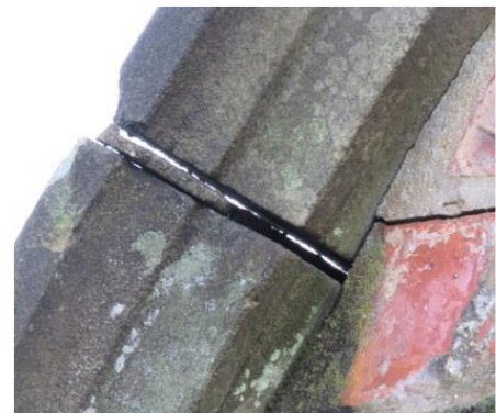
Open joints to gable parapet capping stones.
