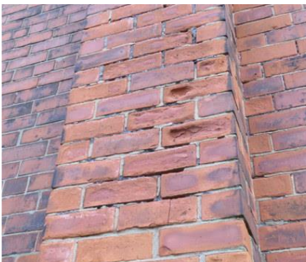
Spalled bricks and open joints to chimney.
