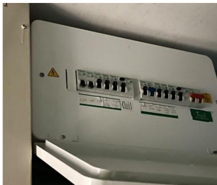
Main electrical board tripped during survey.
