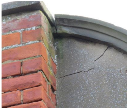
Cracking to high level render to chimney.
