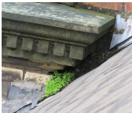
Plant growth in flashings behind gables.
