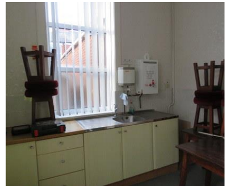
Kitchen dated, water heating dilapidated.
