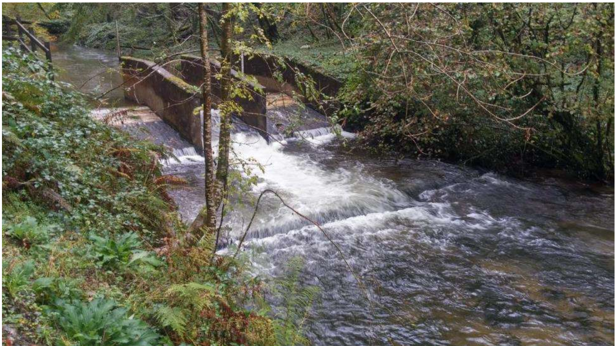
Photo 4: View of structure and downstream pre barrage and eel pass in elevated flows.
