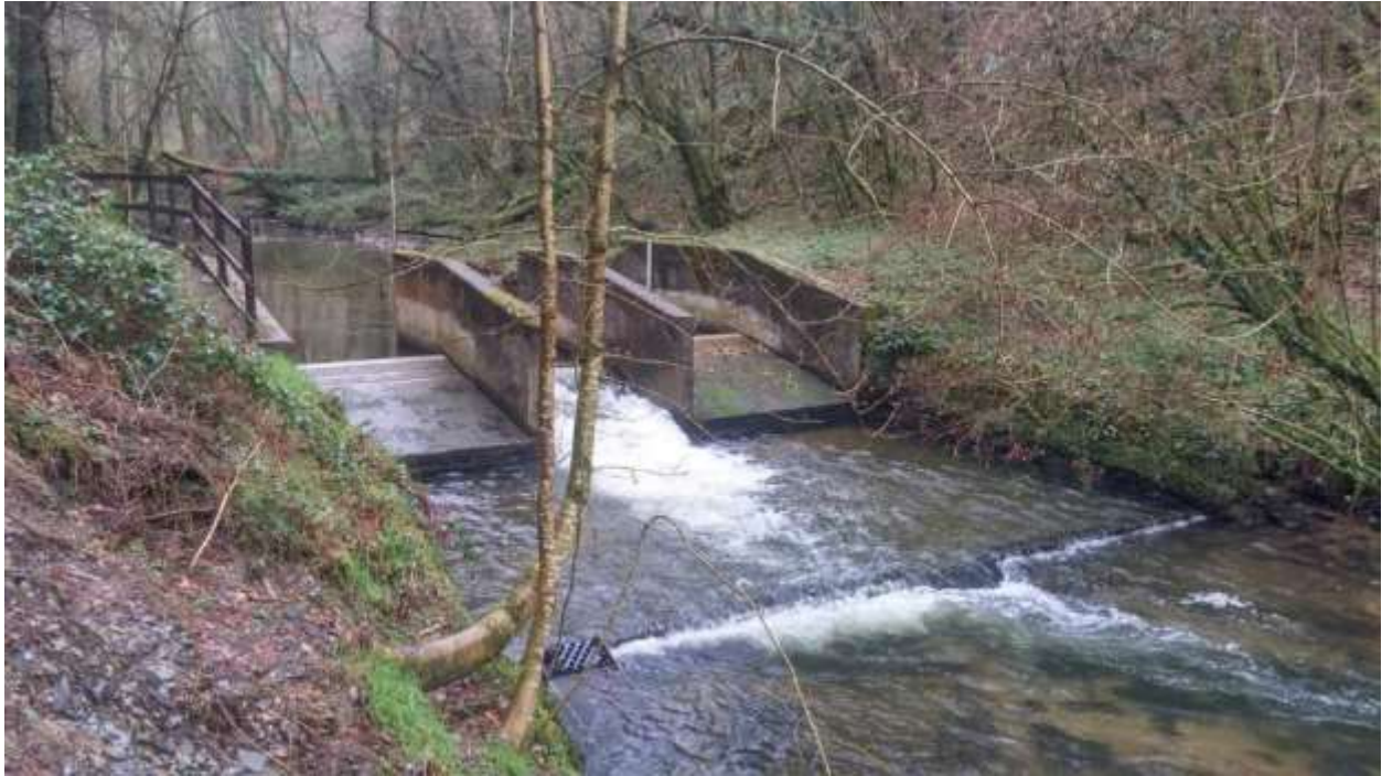
Photo 3: View of structure and downstream pre barrage and eel pass in low flows.
