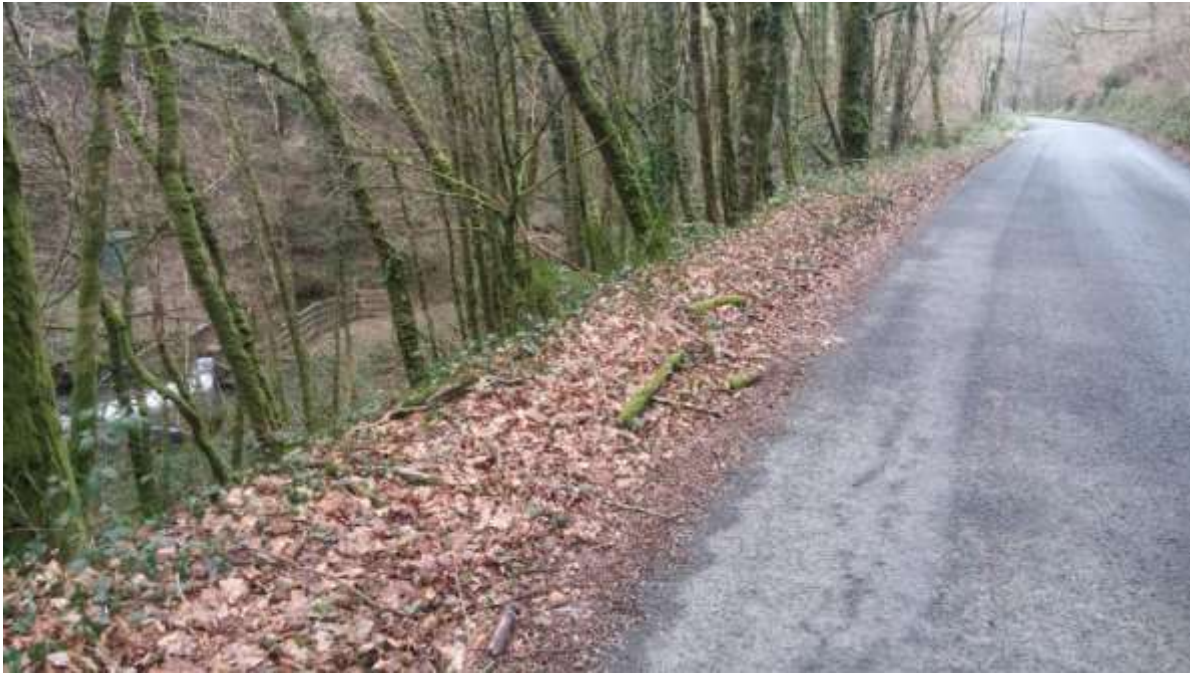
Picture 9: Road adjacent to structure on left hand bank which leads to forestry access gate.
