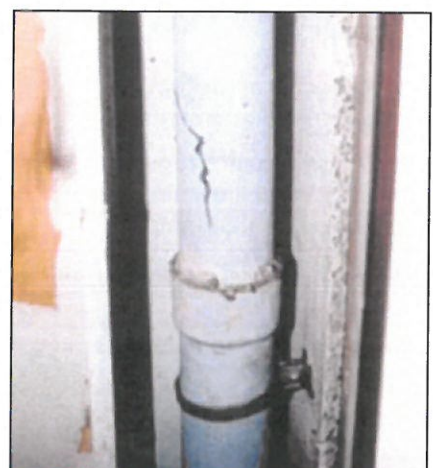
Sometimes the joints are sealed with asbestos string
