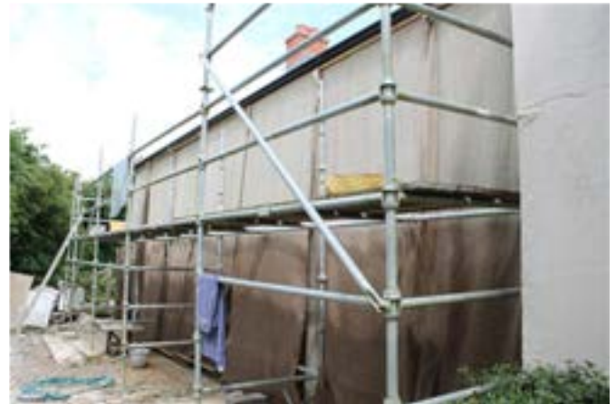
General view of hessian sheeting attached to the inner uprights of a typical inside board scaffolding. Summer working with the hessian dampened down to aid the curing regime.
