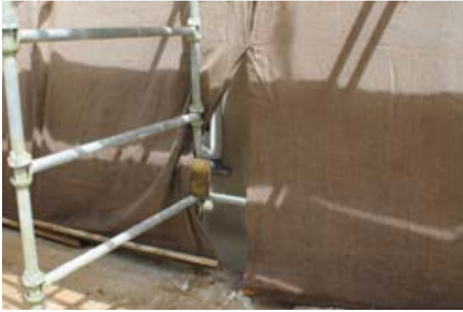
A simple yet effective arrangement at the base of scaffolding to manage hessian protection for a new lime render, note the use of a scaffold board and the 2"x1" batten to mitigate flapping.
