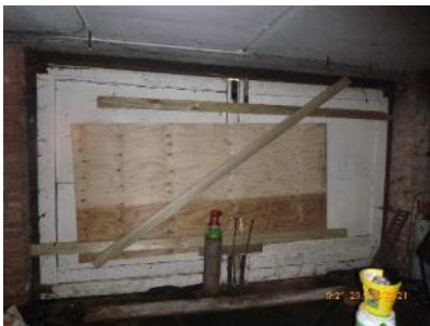
Figure 13. Cellar garage door with gaps around edges.
