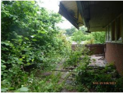
Figure 1. Overgrown terrace hardstanding (paving).
