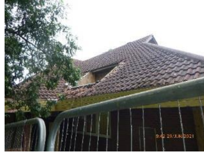
Figure 18. Showing damage around the inverted dormer window on the northern aspect.
