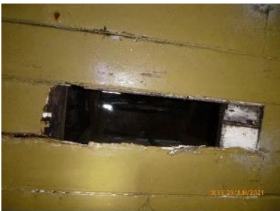
Figure 21. Example of damage to the boarding of the overhanging eaves.
