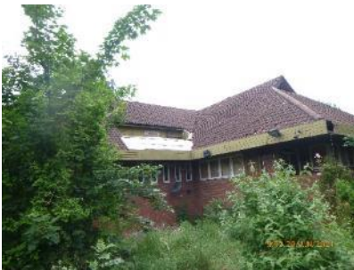
Figure 19. Damage to the roof structure around the inverted dormer leading out from the living kitchen on the southern aspect. Note small section of weatherboarding where roof sections meet.
