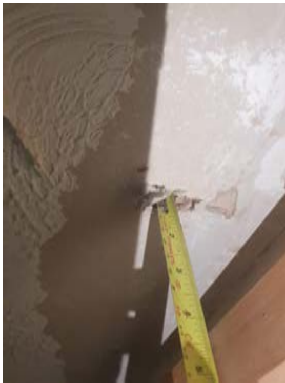
Photo098 – B05 - Basement Room 3 - 25mm depth of Plasterboard to ceiling.
