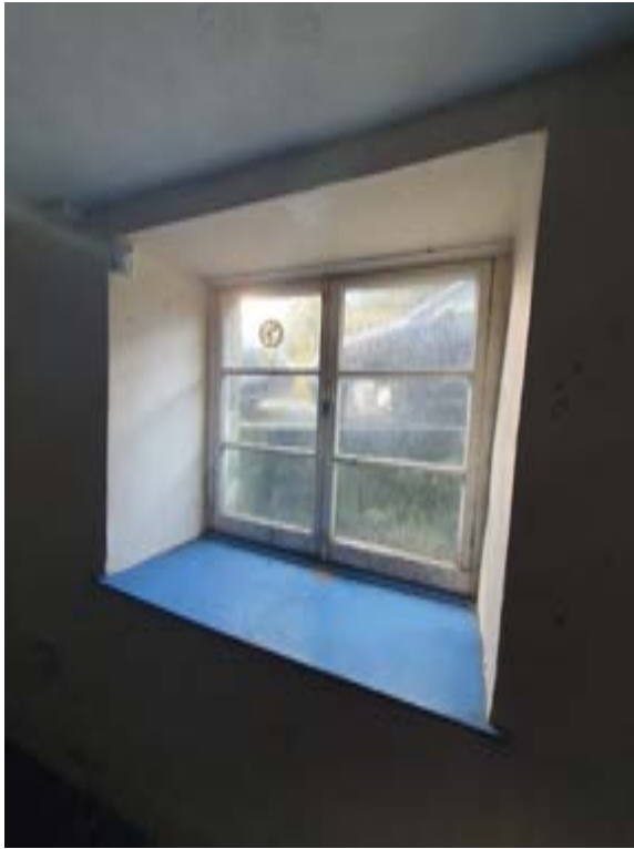
Photo065 – B04 - Basement Room 2 - Window WB1
