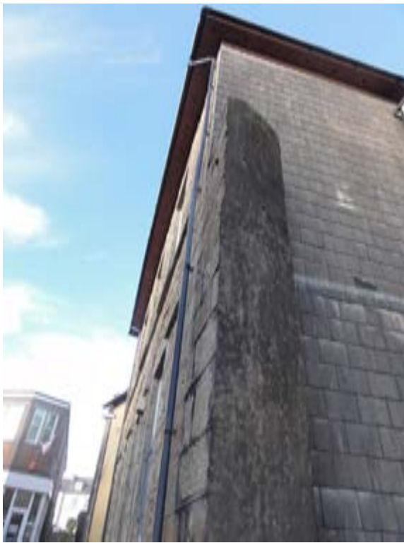
Photo385 – External - Possible Asbestos Hung Slate, damage to be repaired - Party Wall
