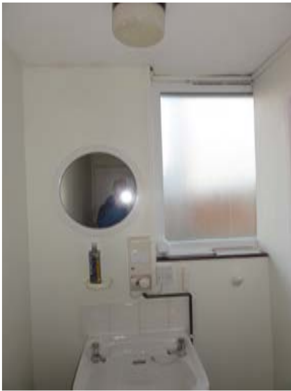
Photo297 – G11 - WC 3 - Window WG2. Layout to be reconfigured.
