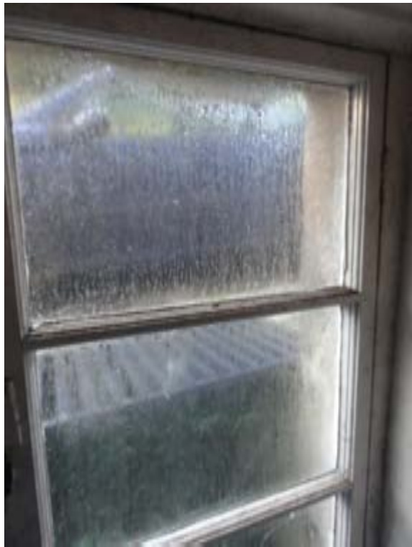
Photo064 – B04 - Basement Room 2 - Window WB1
