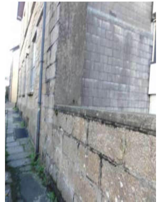
Photo384 – External - Possible Asbestos Hung Slate, damage to be repaired - Party Wall
