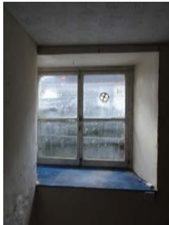
Photo100 – B05 - Basement Room 3 - Window WB3
