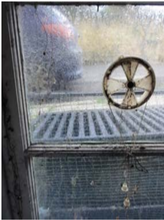
Photo089 – B04 - Basement Room 2 - Window WB2
