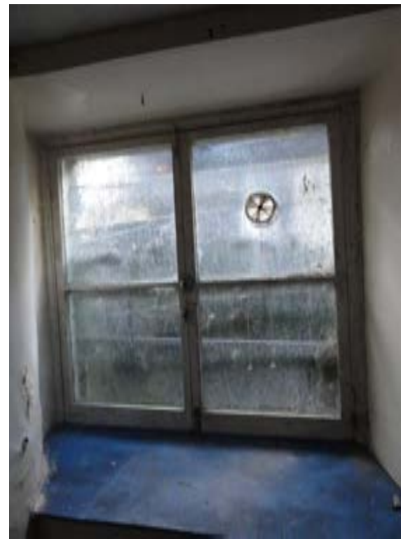
Photo102 – B05 - Basement Room 3 - Window WB3
