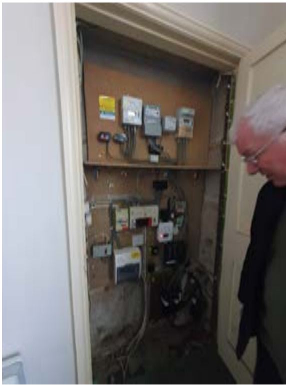
Photo121 – G01 - Office 1 - 3 Phase Power CPD. Door DG5
