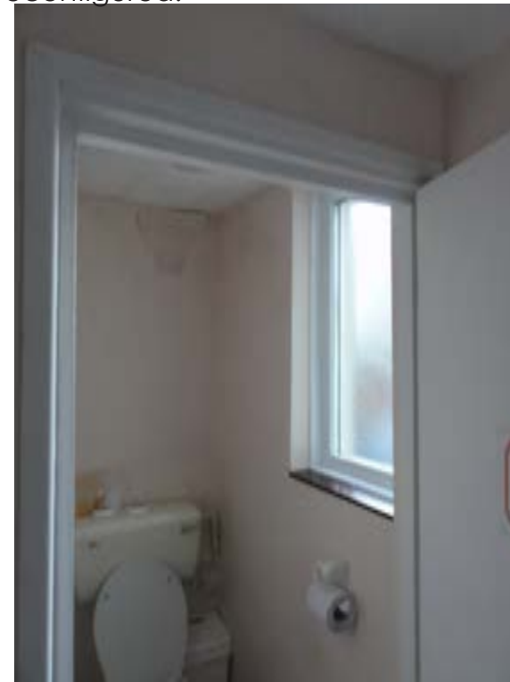
Photo294 – G10 - WC 2 - Window WG3 and Door DG26 (To be removed). Layout to be reconfigured.
