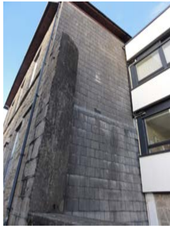
Photo387 – External - Possible Asbestos Hung Slate, damage to be repaired - Party Wall
