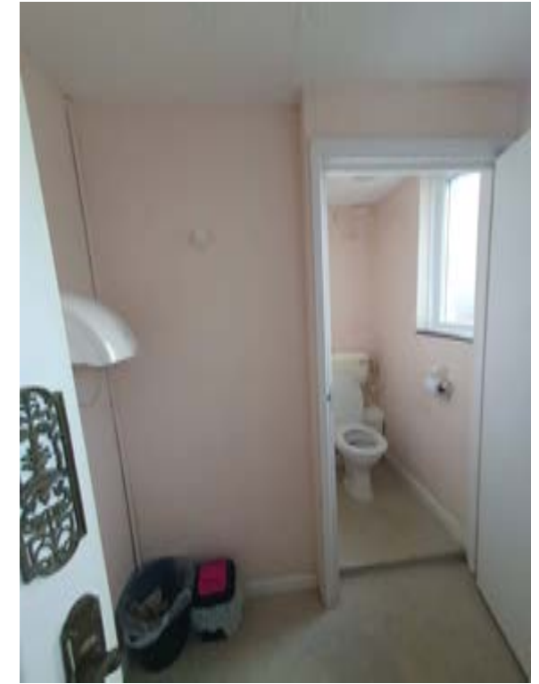
Photo295 – G10 - WC 2 - Window WG3 and Door DG26 (To be removed). Layout to be reconfigured.
