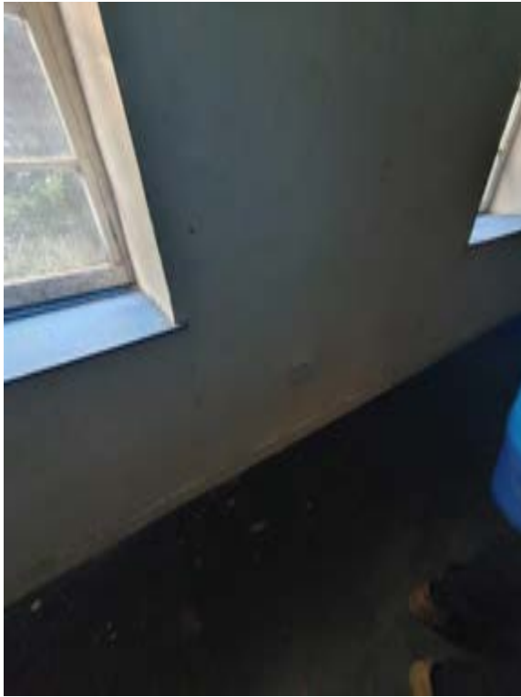
Photo081 – B04 - Basement Room 2 - Window WB1
