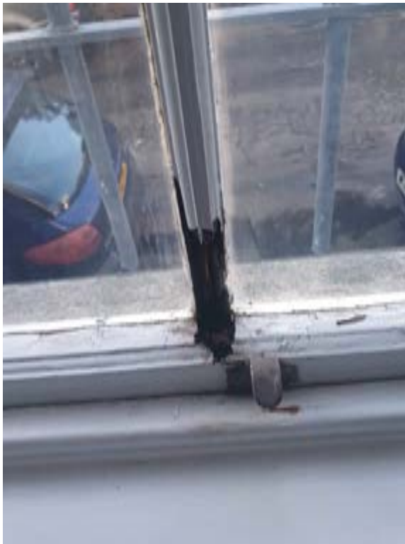
Photo226 – G04a - Lobby - Window WG7 bottom sash damaged and needs repairing.
