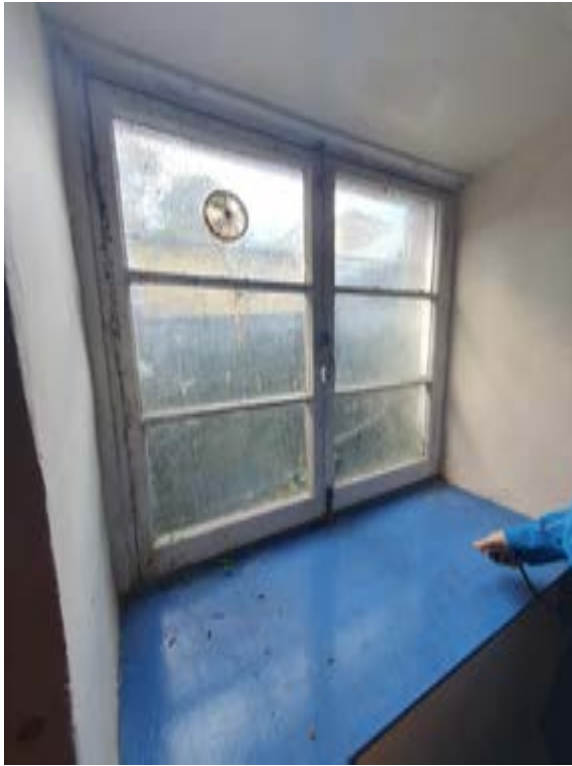
Photo073 – B04 - Basement Room 2 - Window WB2
