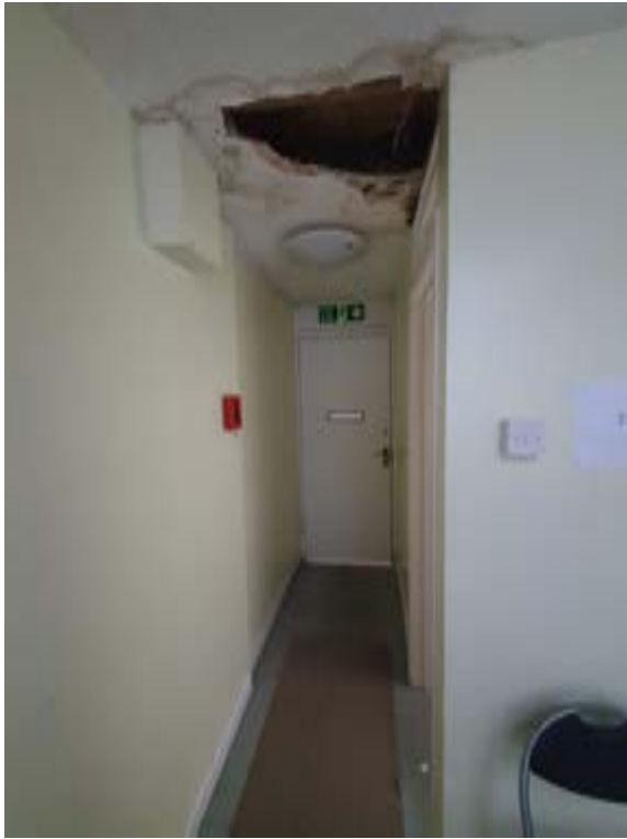
Photo273 – G07 - Kitchen 1 - Door DG11 - Ceiling repair needed.
