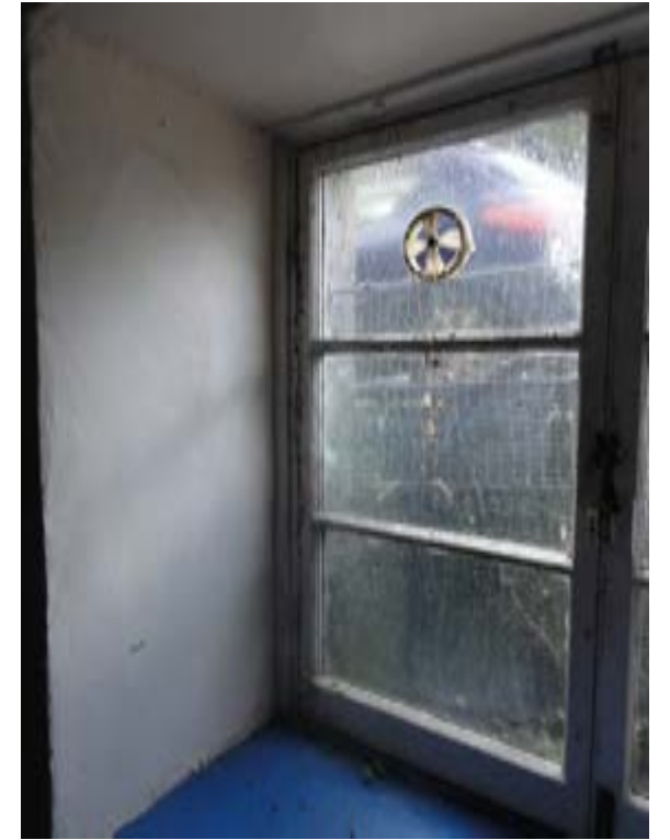
Photo087 – B04 - Basement Room 2 - Window WB2
