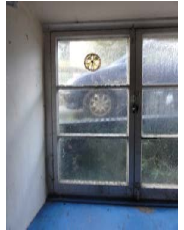
Photo088 – B04 - Basement Room 2 - Window WB1
