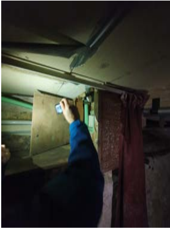
Photo049 – B03 - Basement Room 1 - Water Meter CPD.
