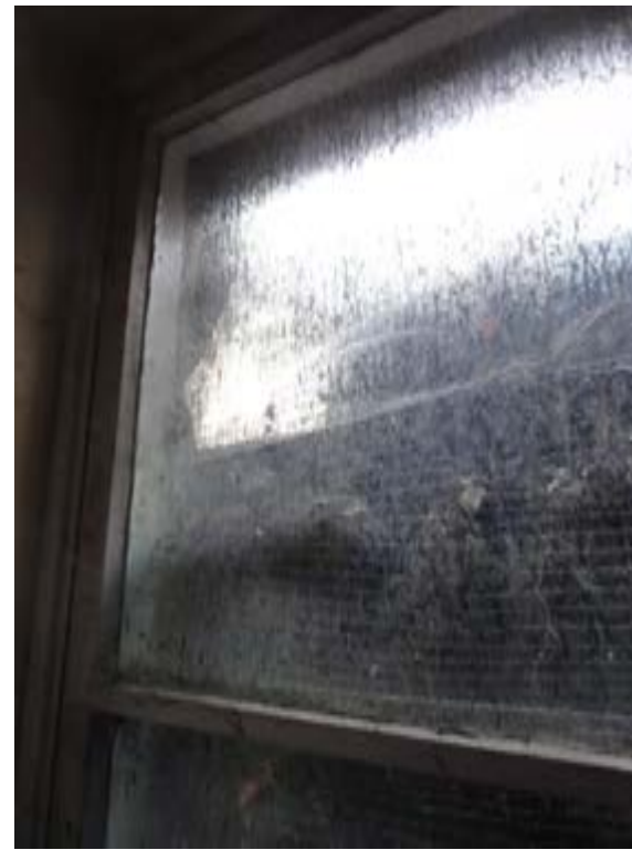
Photo093 – B05 - Basement Room 3 - Window WB3
