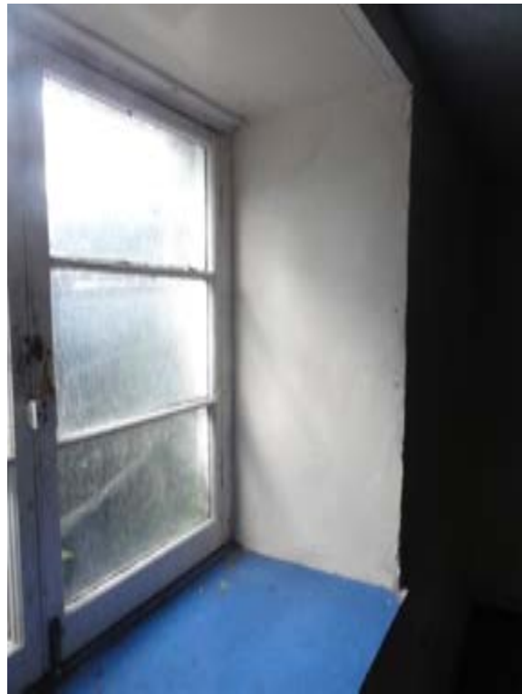
Photo084 – B04 - Basement Room 2 - Window WB2
