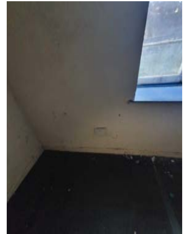
Photo080 – B04 - Basement Room 2 - Window WB1
