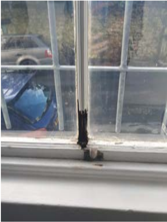
Photo231 – G04a - Lobby - Window WG7 bottom sash damaged and needs repairing.
