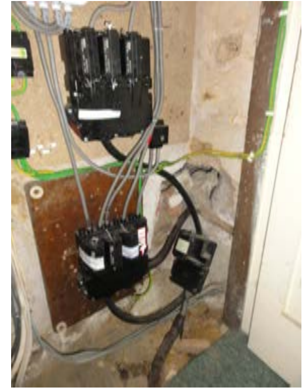
Photo135 – G01 - Office 1 - 3 Phase Power CPD. Door DG5
