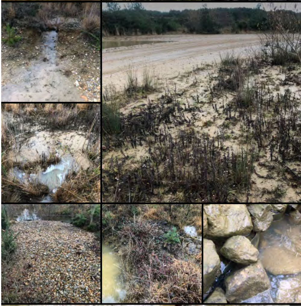
Evidence of turbid/sandy runoff from track but good functioning of check dam with lower turbidity downstream
