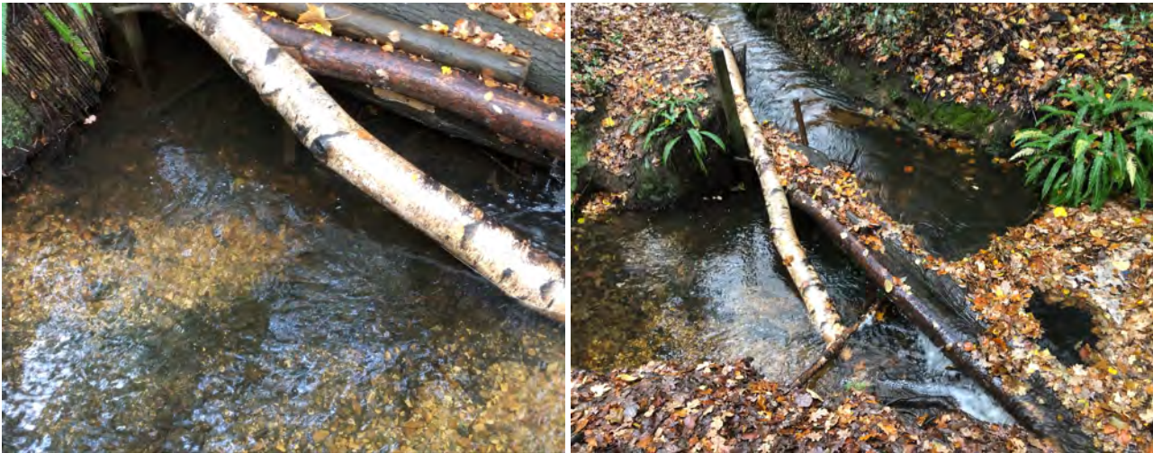
Plates 3 and 4. Leaky woody dam and flow passing below the structure but majority of flow passing down the diversion channel.
