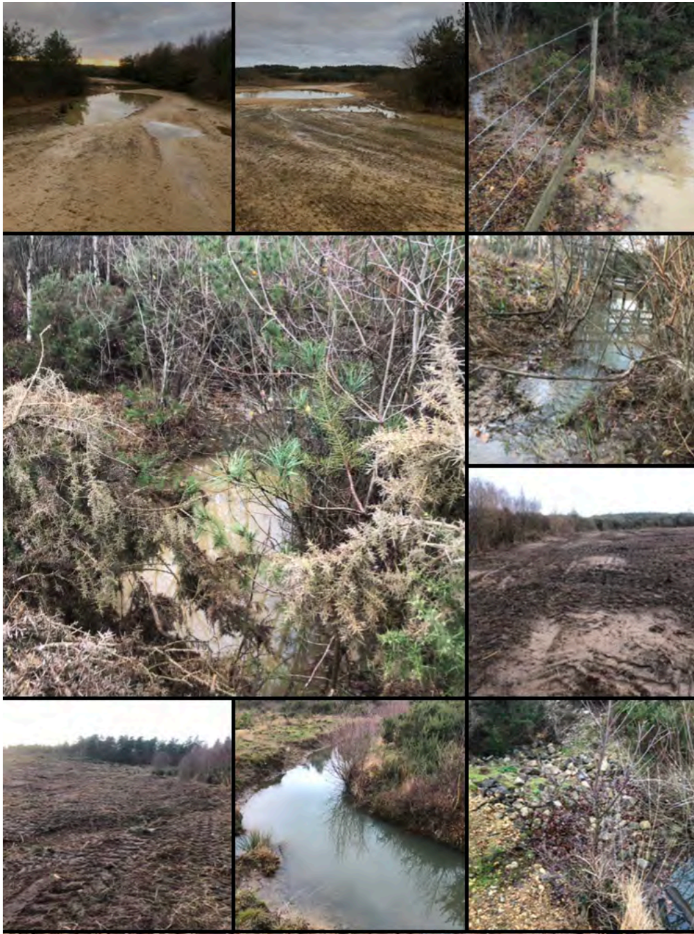
Eroding tracks and channels close to the lower balancing/holding lagoon and adjacent heath management works. Improved turbidity below lagoon.
