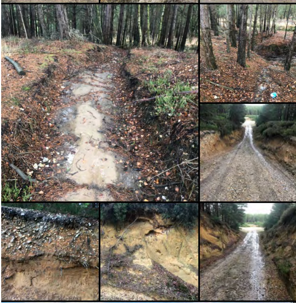
Stable gully tracks with new runoff channel and some sandy erosion
