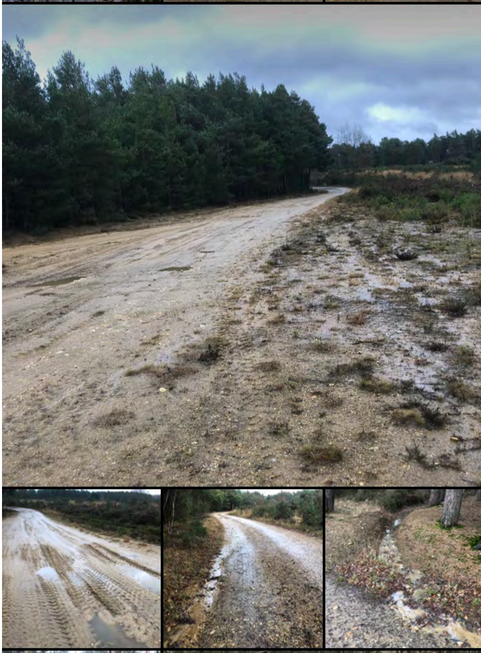
The outer tracks show evidence of surface water flow and sediment transport although this continues to be diverted across the track into an adjacent setline/management pond.
