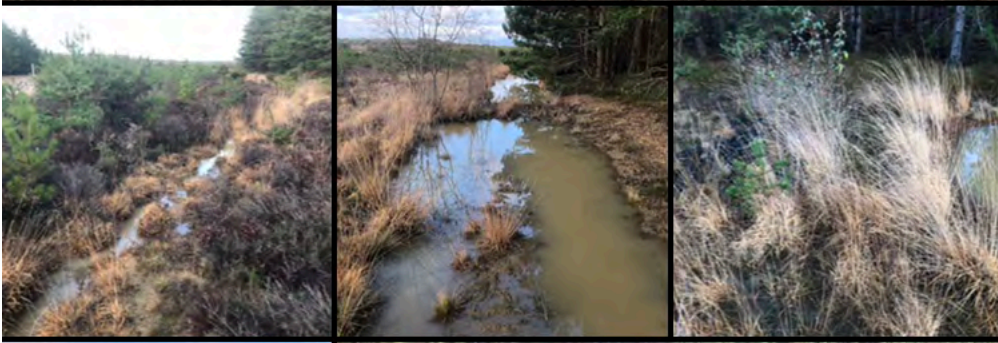
Continued functioning of diversion feature pushing turbid and sandy flow into marginal habitats and channel
