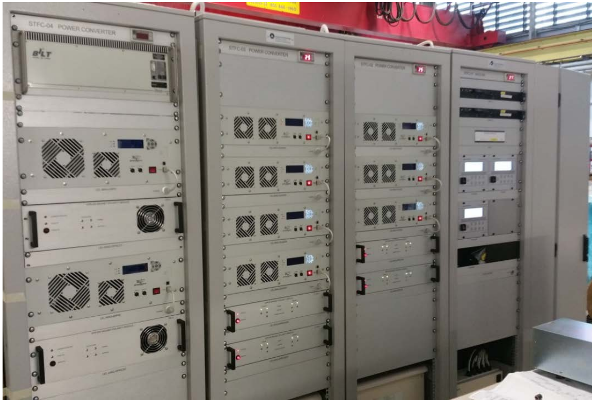
Figure 2: Power supply, controls & Instrumentation Racks
