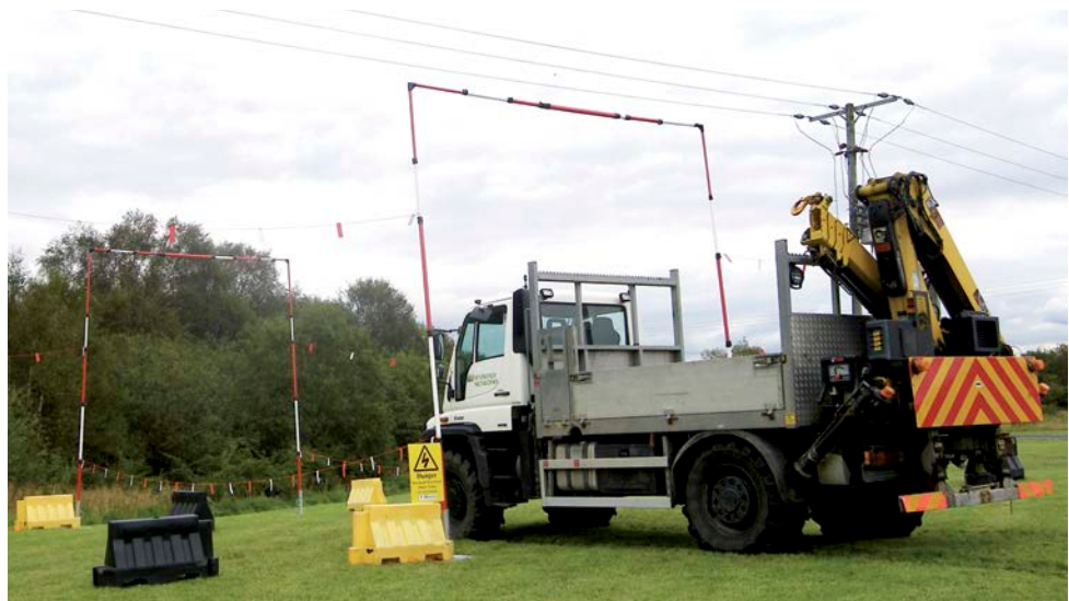
Figure 5 Typical passageway through barriers
