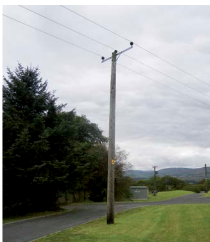
Figure 2 11 kV distribution line
