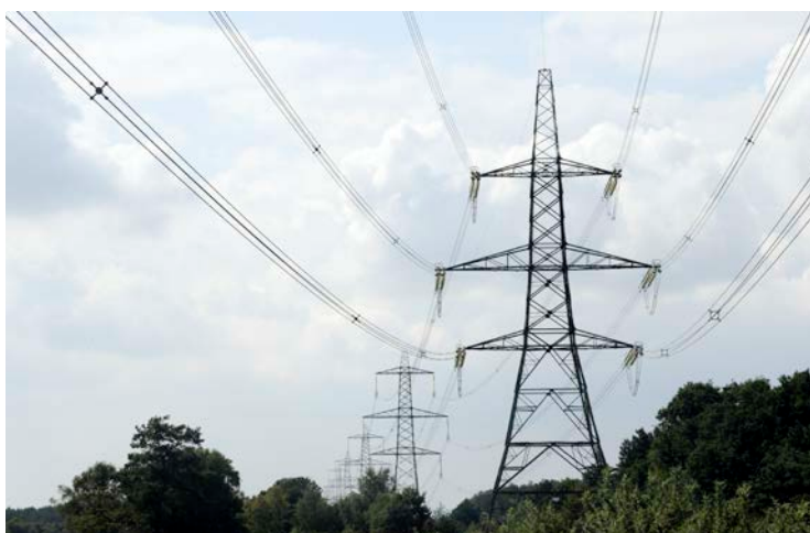
Figure 1 275 kV transmission line
