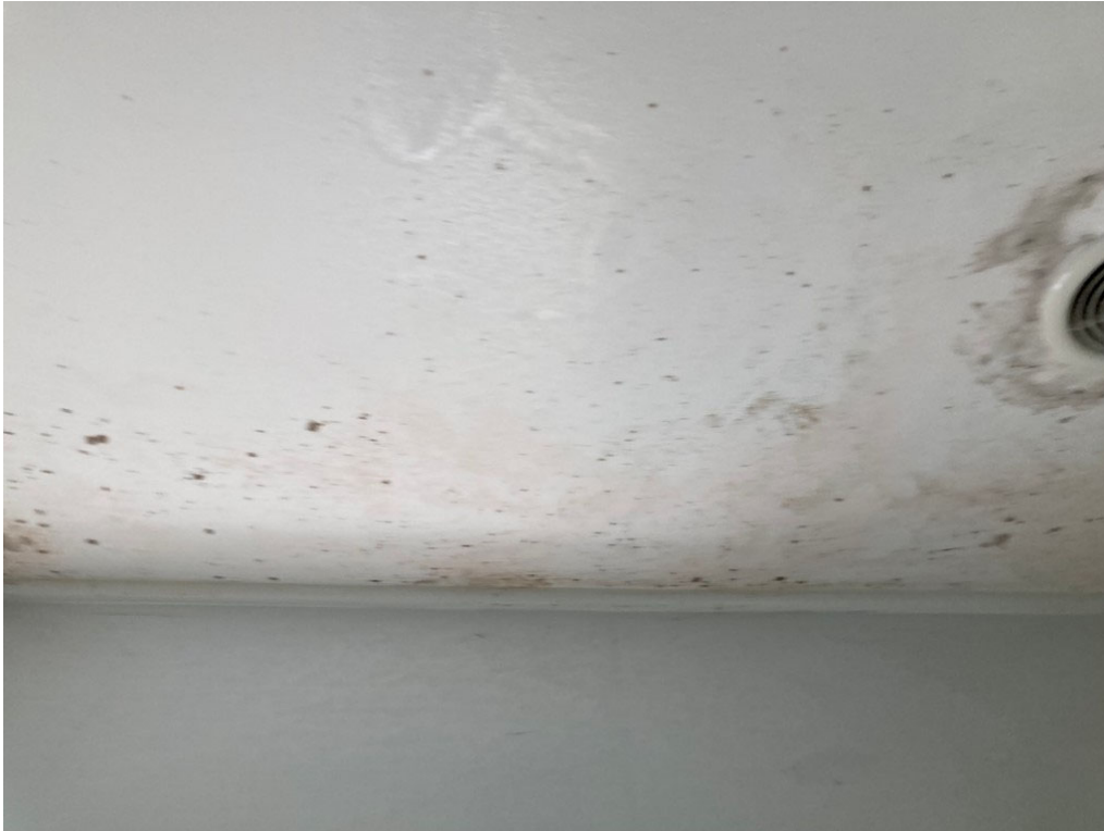
Mould growth in bathroom (2)
