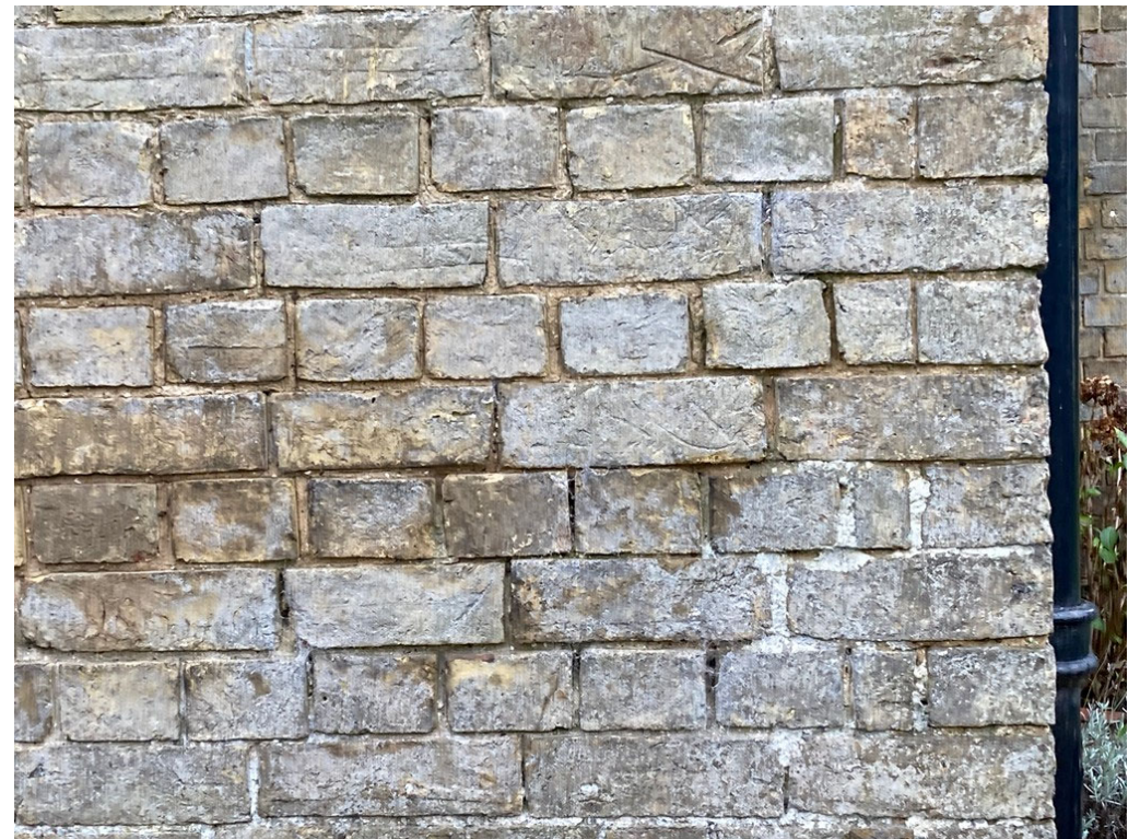
Example of area in need of repointing
