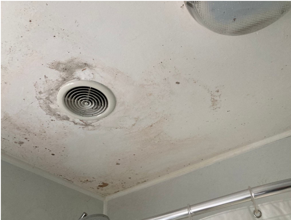
Mould growth in bathroom
