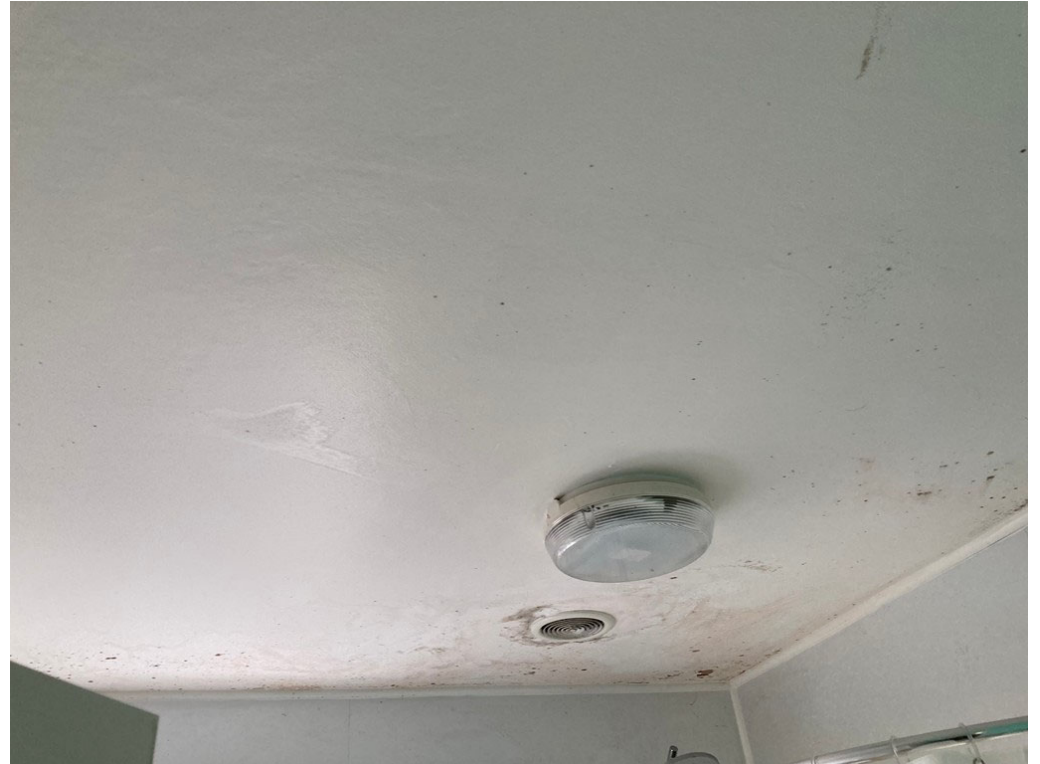
Mould growth in bathroom (3)
