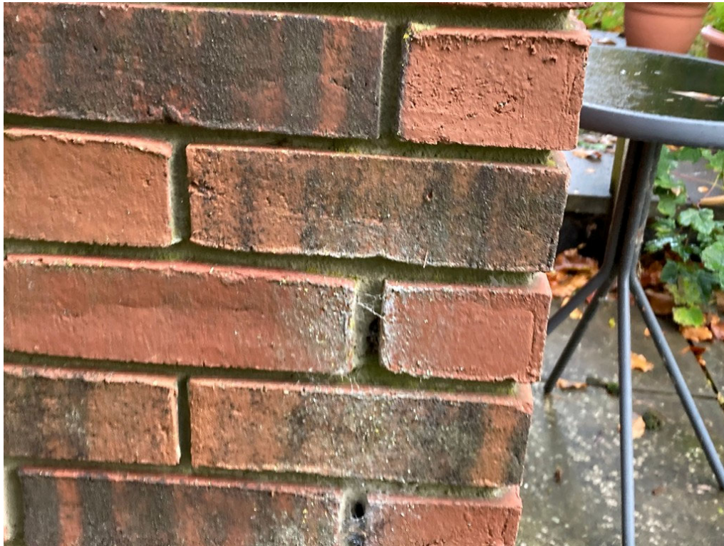
Example of area in need of repointing
