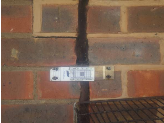
7. Wall 1 Crack monitoring gauge suggesting 4mm vertical movement
