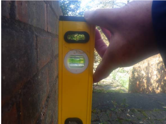
37. Wall B Leaning out of vertical
