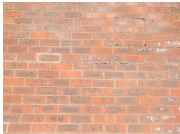
24. Wall 7 Very slightly tapering vertical fracture
