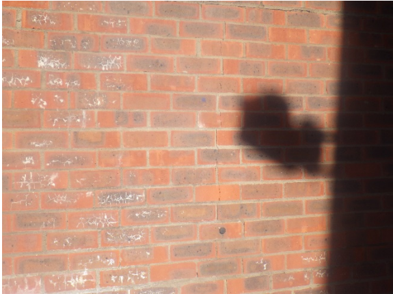
25. Wall 7 Very slightly tapering vertical fracture
