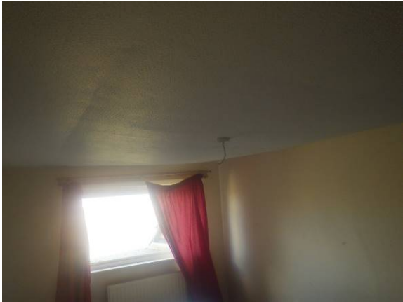
18. Sagging ceiling to first floor Bed 1
