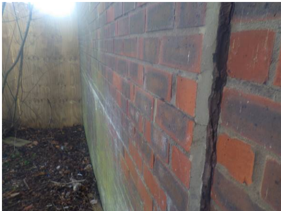
33. Wall A No weep holes
