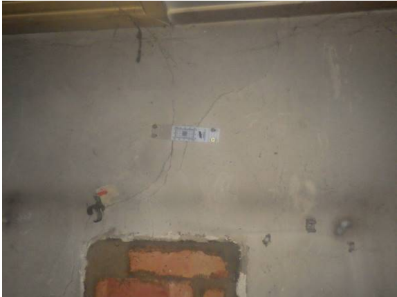
14. Crack monitor to Wall 1 suggesting no significant movement recorded
