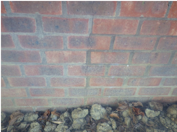
30. Wall 12 continuation of fracture in photo 29.
