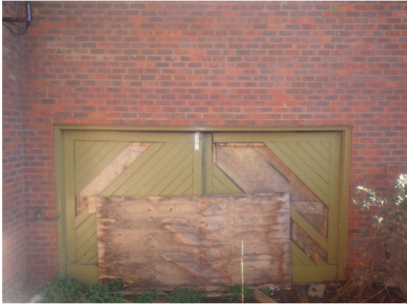
26. Wall 8 showing very slight sag to door head
