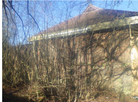
38. Wall B Rear face also showing dense vegetation
