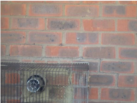
6. Wall 1 Stepped fracturing above vent grill
