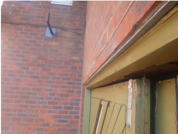
28. Wall 8 Slight lateral displacement in brickwork over
