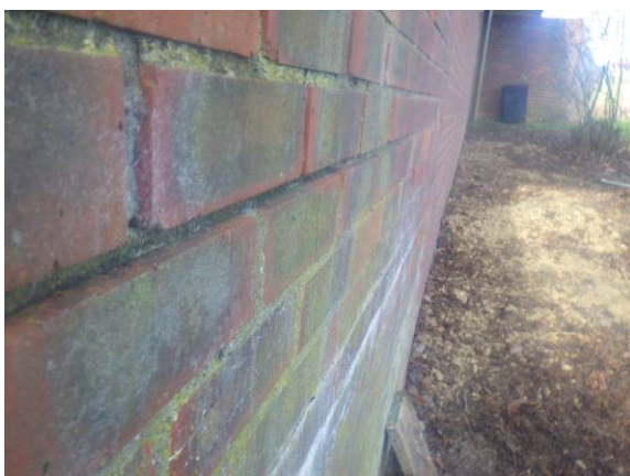
35. Wall A 5mm lateral displacement at dpc level
