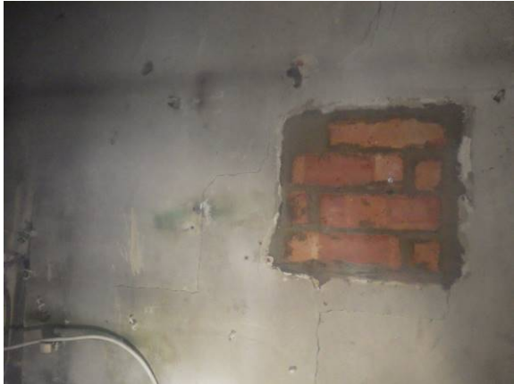
13. Wall 1 fracturing within Boiler room
