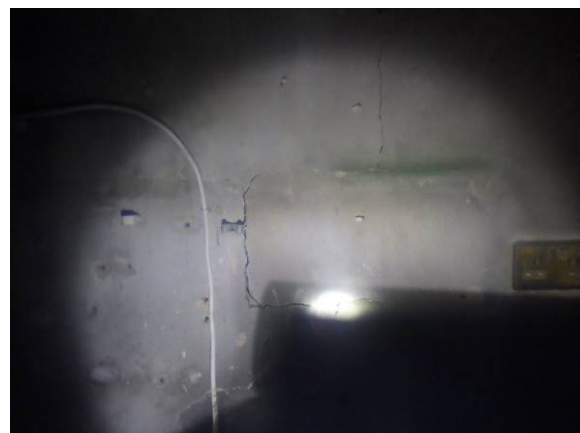
12. Fracturing to Wall 1 within Boiler room
