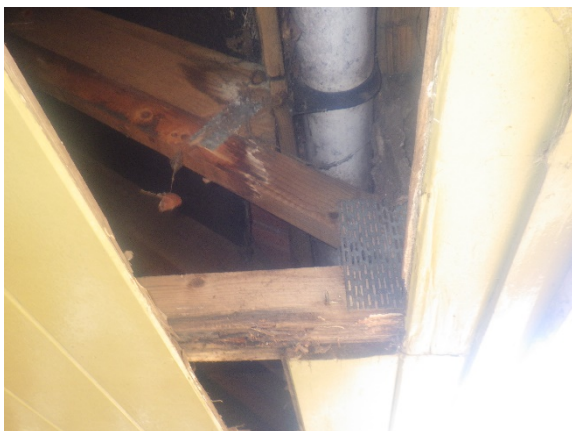
23. Wall 4 Water damage and decay to timbers
