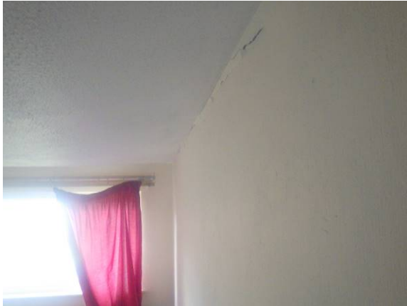
19. Laterally displaced plaster due to ceiling sag in Bed 1
