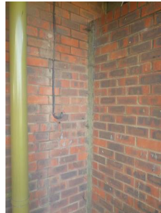
44. Wall D Wide tapering mortar fillet at abutment with building
