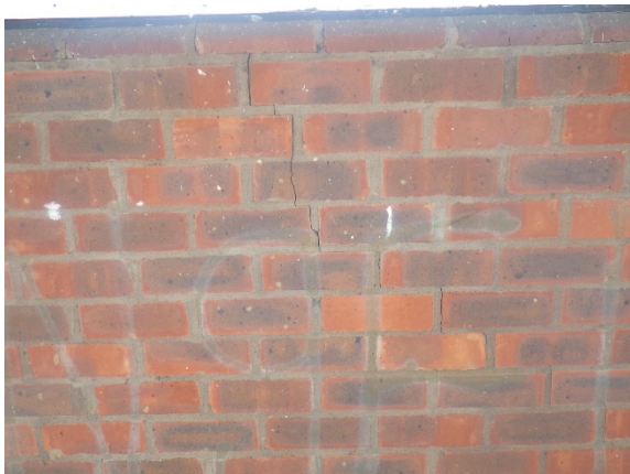
21. Wall 4 slightly tapering width vertical fracture
