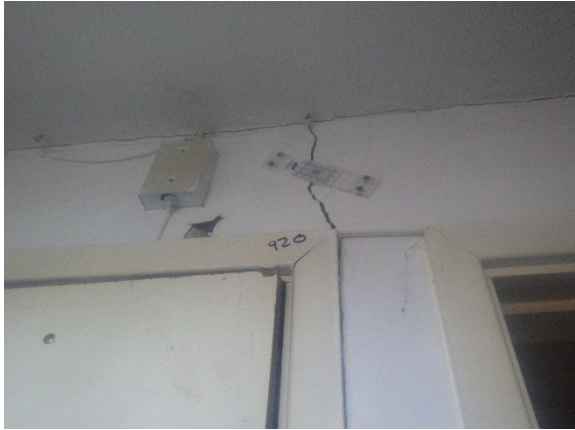
15. Top edge of door binding where frame has dropped
