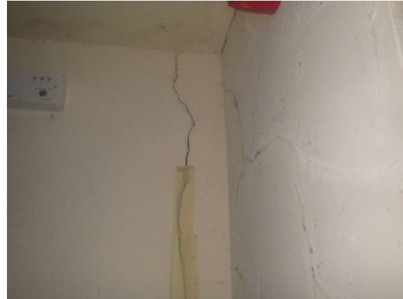
8. Fracture to corner of Disabled WC dividing wall with Boiler room
