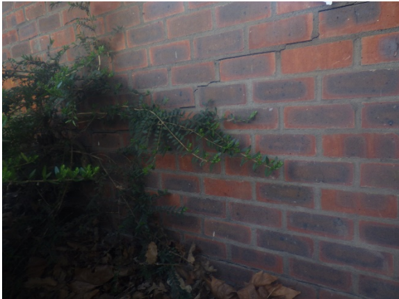
3. Wall 1 horizontal and diagonal stepped fracturing and adjacent shrubs
