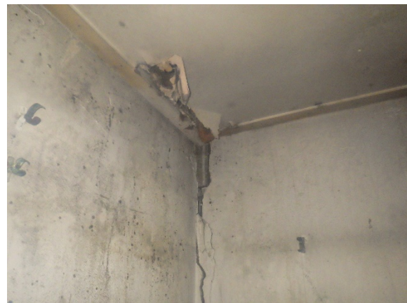
10. Fracture reflected within Boiler room dividing wall with Disabled WC at rear of stairwell, also showing beading at ceiling junction.
