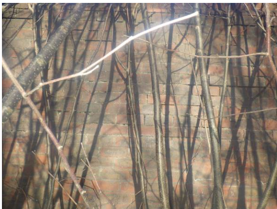
39. Wall B Rear face open joints, no weep holes
