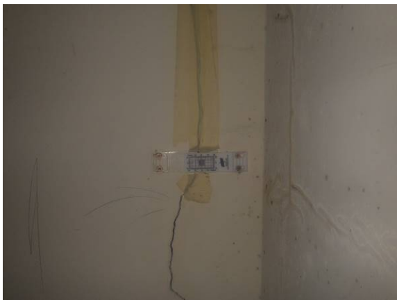
9. Fracture to corner of Disabled WC dividing wall with Boiler room indicating the wall to the left has lifted in the region of 4mm
