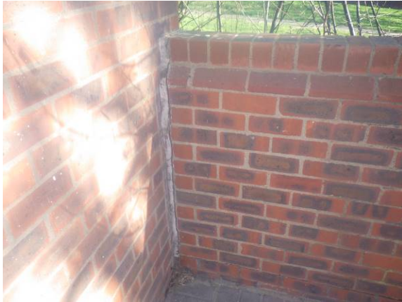
31. Wall A displacement
