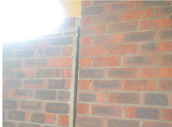
32. Wall A displacement
