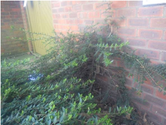
4. Wall 1 horizontal and diagonal stepped fracturing and adjacent shrubs
