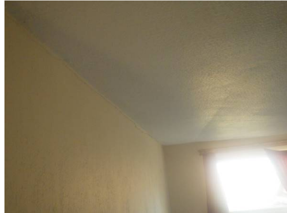
20. Laterally displaced plaster due to ceiling sag in Bed 1
