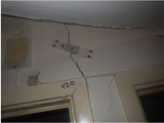
16. Crack monitor to adjacent room suggesting no significant movement recorded
