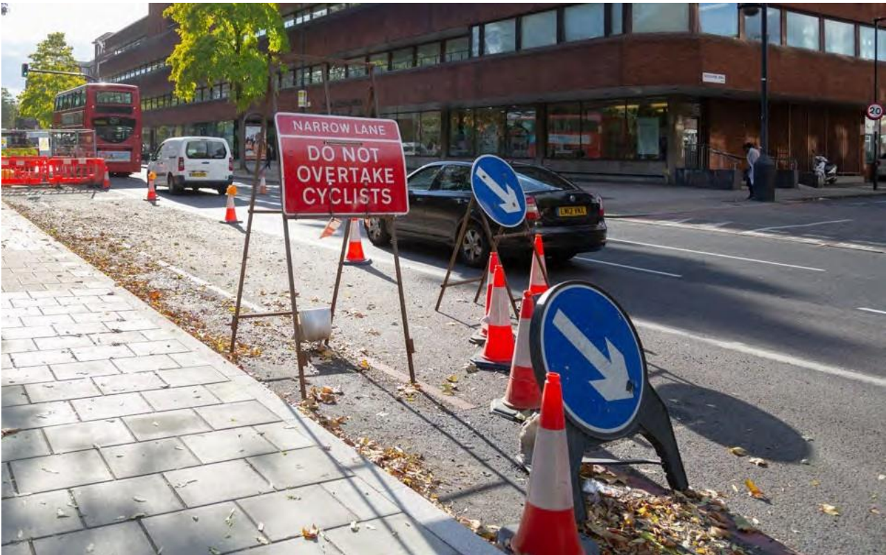
Correct warning sign
