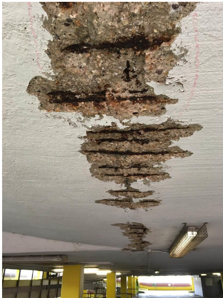
Figure 6: Multiple areas of spalling to soffit throughout car park, exposing corroded reinforcement bars.
