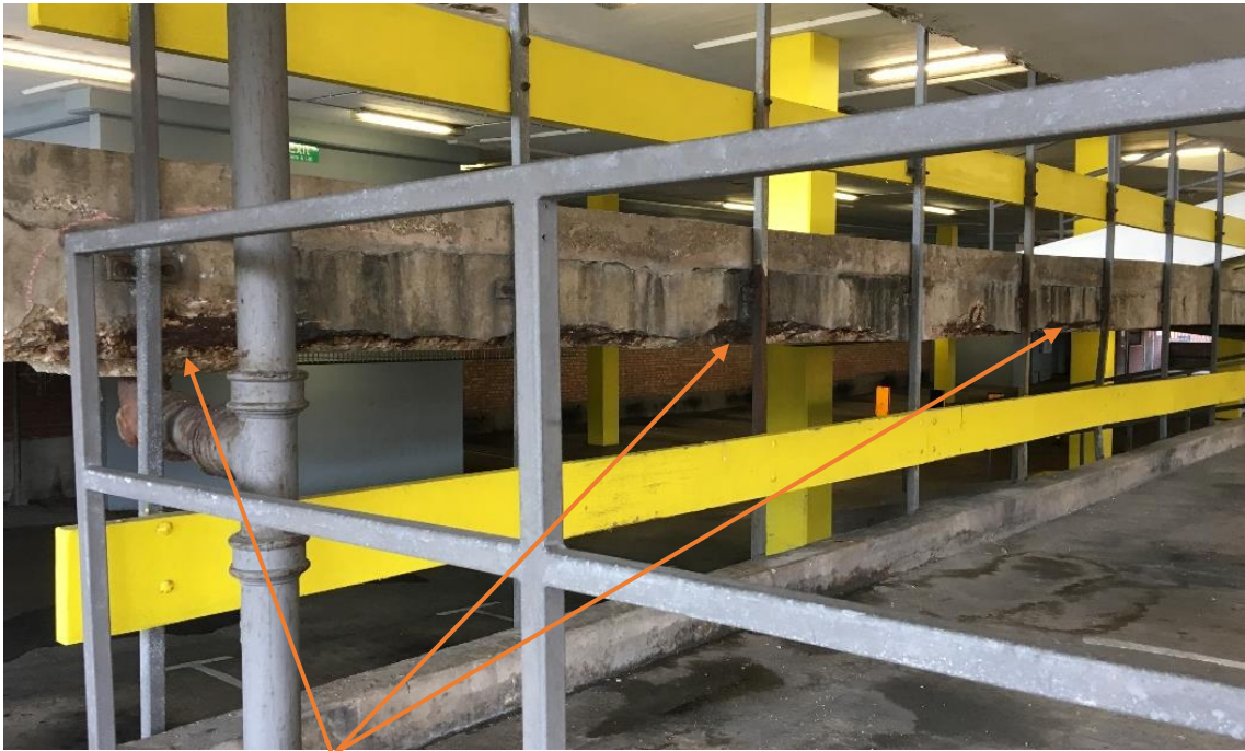
Figure 5: Spalling to concrete exposing corroded reinforcement bars at edge of deck.
