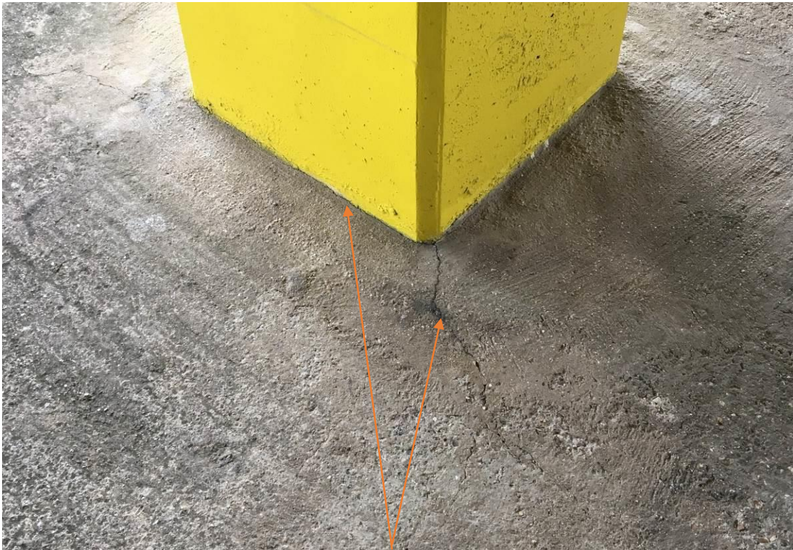
Figure 3: Fresh cracking through repair material around base of column, crack <2mm wide.
