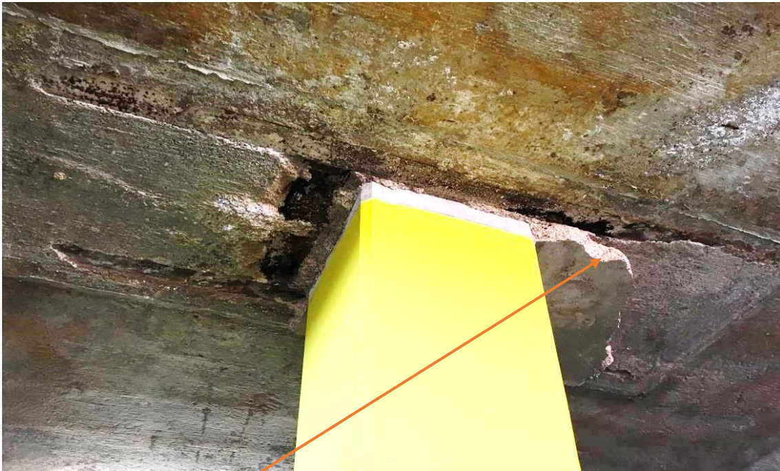
Figure 1: Spalled concrete protection around column exposing corroded steel collar.
