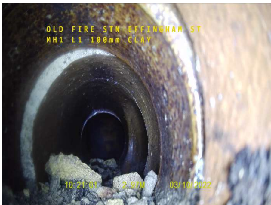
Photo: 1_1_7_A.jpg 3.07m, Joint displaced, medium
