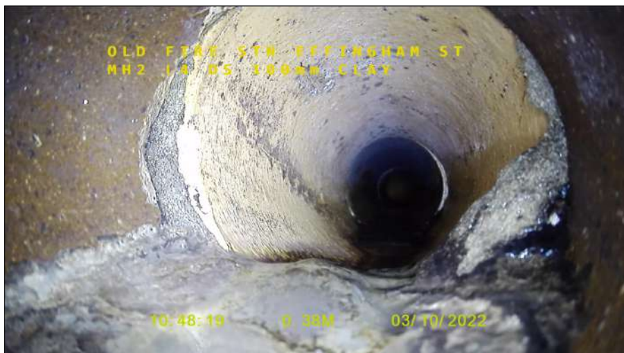
Photo: 11_11_57_A.jpg 0.28m, Settled deposits, hard or compacted at joint, 10% cross-sectional area loss
