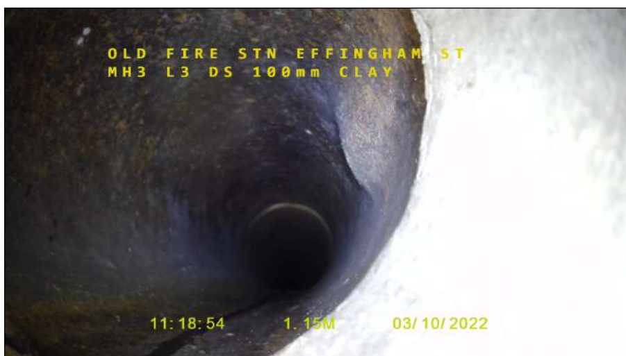
Photo: 14_14_97_A.jpg 1.15m, Deformed sewer/drain, 5%
