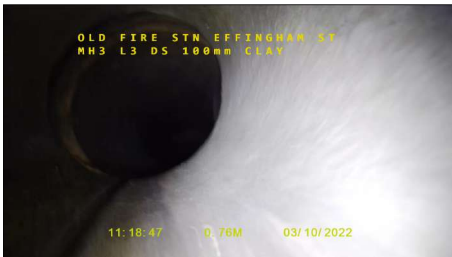
Photo: 14_14_96_A.jpg 0.96m, Joint displaced, medium
