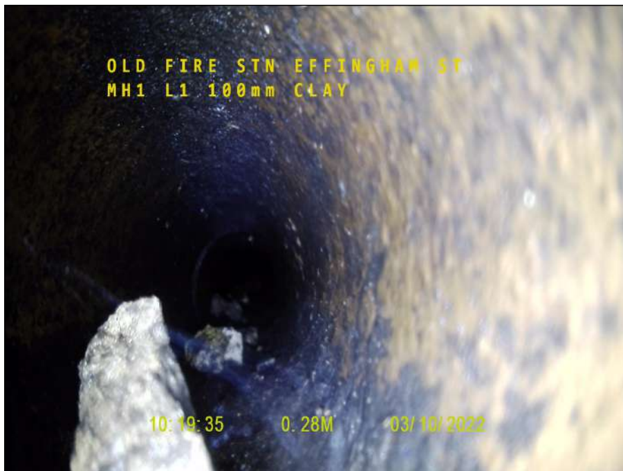
Photo: 1_1_4_A.jpg 0.28m, Settled deposits, coarse, 10% cross-sectional area loss, Start
