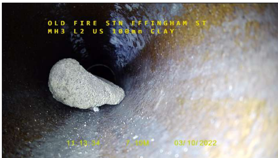
Photo: 13_13_90_A.jpg 7.01m, Settled deposits, coarse, 30% cross-sectional area loss
