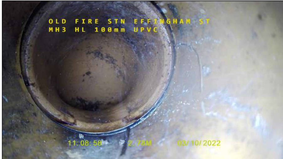
Photo: 12_12_86_A.jpg 2.97m, Finish node type, gully reference number: RWP
