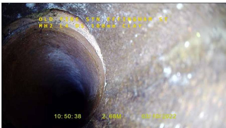
Photo: 11_11_63_A.jpg 2.68m, Joint displaced, medium
