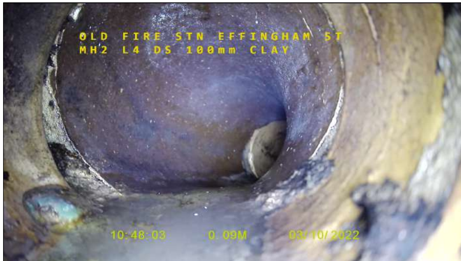
Photo: 11_11_54_A.jpg 0.1m, Joint displaced, medium
