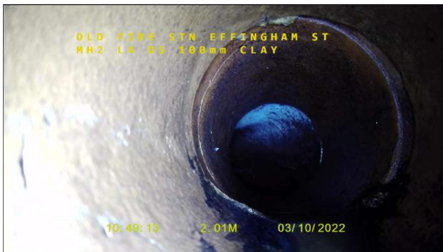
Photo: 11_11_61_A.jpg 2.01m, Crack, circumferential at joint, from 7 to 12 o'clock
