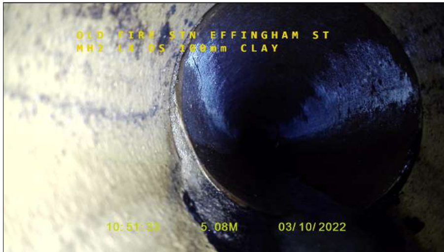
Photo: 11_11_68_A.jpg 5.08m, Joint displaced, medium
