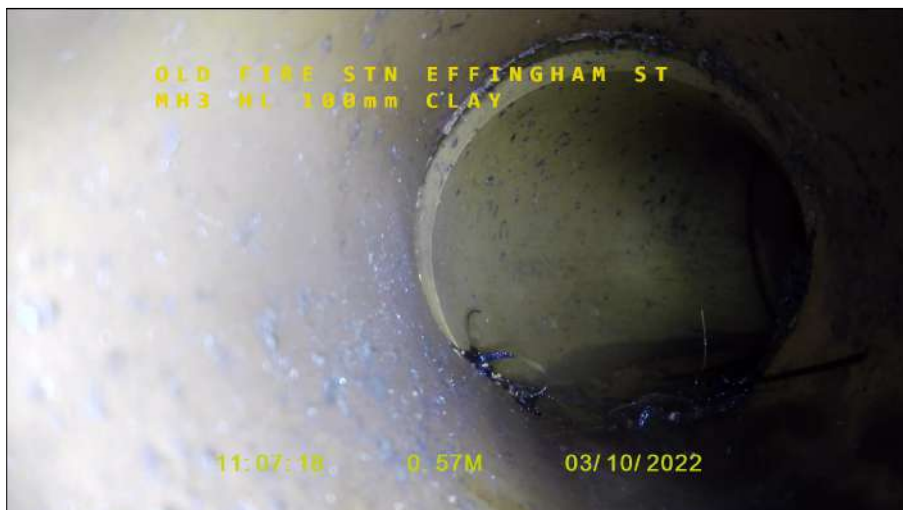
Photo: 12_12_83_A.jpg 0.67m, Roots, fine at joint
