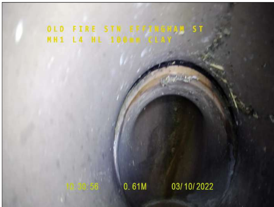
Photo: 5_5_24_A.jpg 0.61m, Joint displaced, medium
