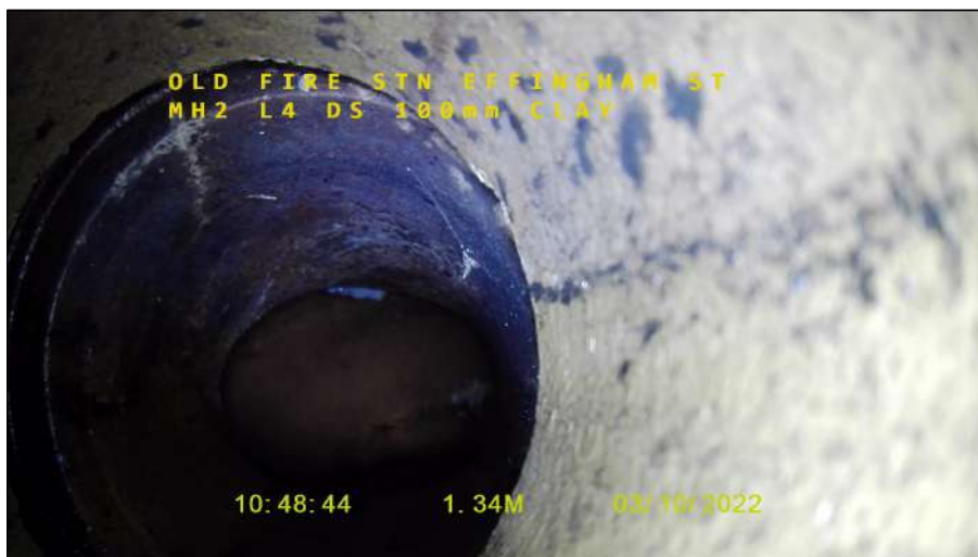
Photo: 11_11_59_A.jpg 1.34m, Joint displaced, medium
