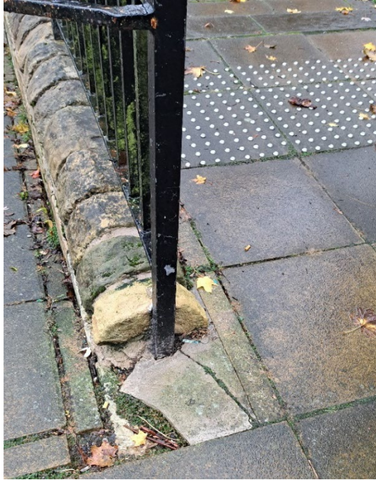
Figure 10 View of current damage to end of wall adjacent to railings
