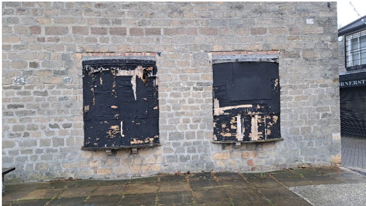
Figure 12 View of the boarded former windows to the side gable of 5 Cotton Street
