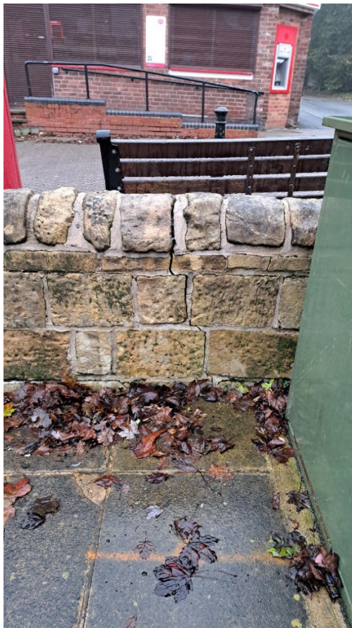
Figure 8 View of crack in wall to north elevation
