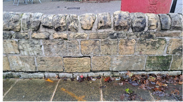
Figure 7 View of crack through wall
