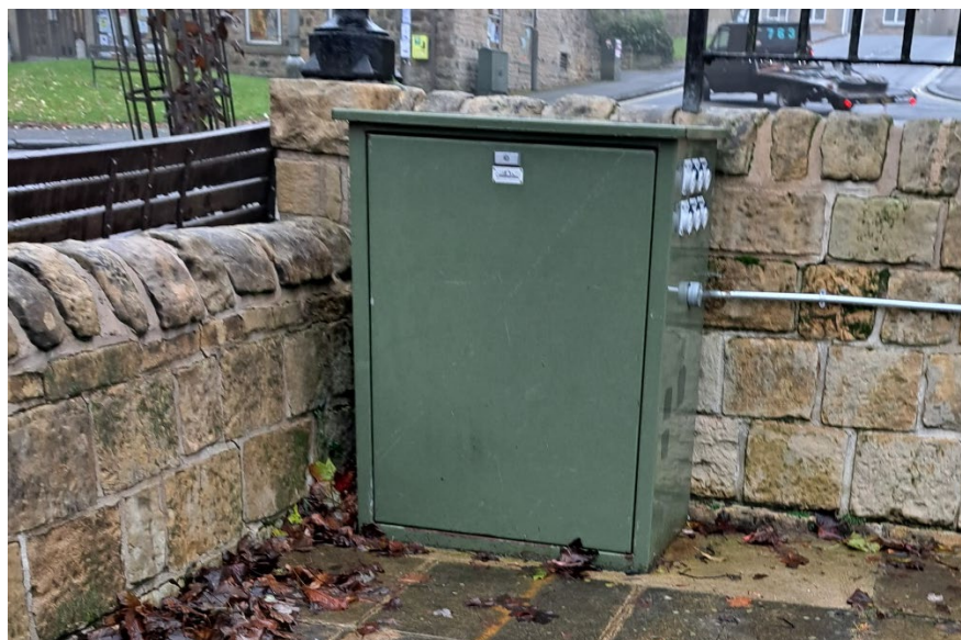
Figure 5 View of existing electrical cabinet
