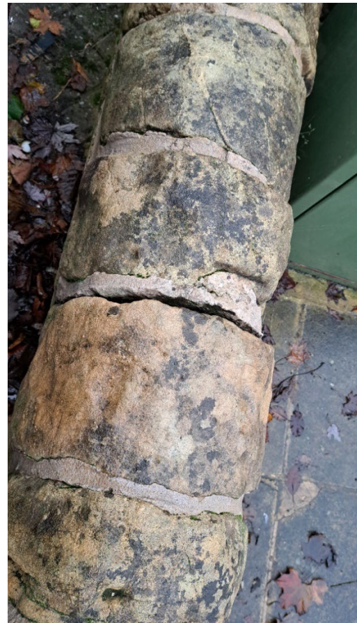
Figure 9 View of crack in wall from above
