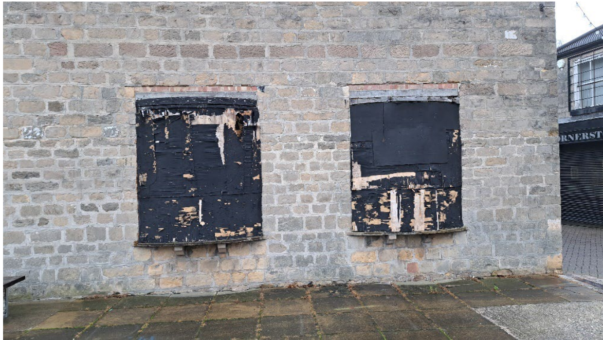
Figure 4 View of the boarded former windows to the side gable of 5 Cotton Street
