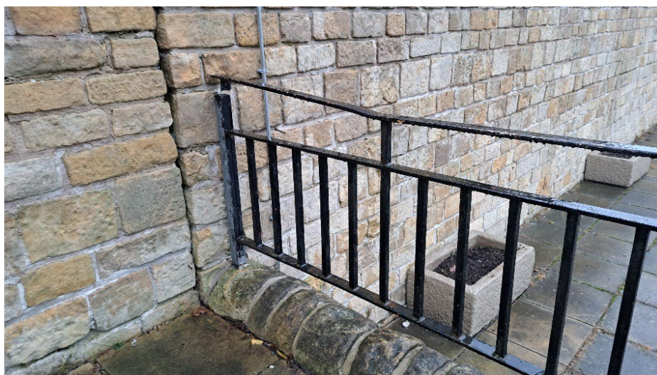
Figure 11 View of current damage to railings at head of ramp
