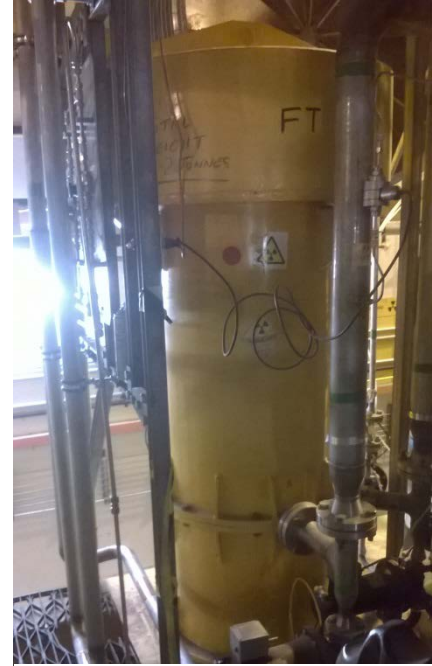
Figure 1 - Existing TS1 Filter Shielding
