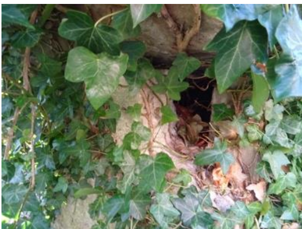
Hole at the top right corner of the east end.
