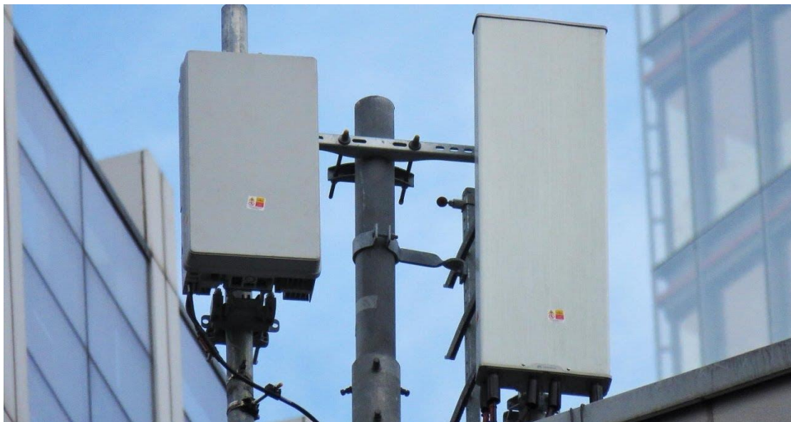
Figure 2: Example of Huawei 5G antenna system
