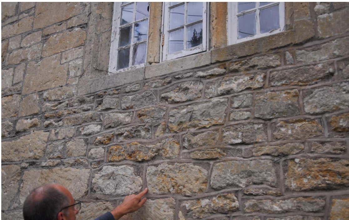
Figure 22 Vertical crack below WF2
