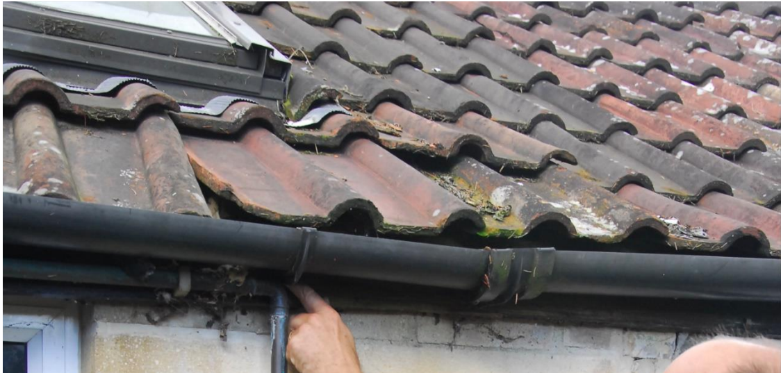
Figure 18 RS 10 Dislodged tiles most likely associated with top plate or rafter end failure
