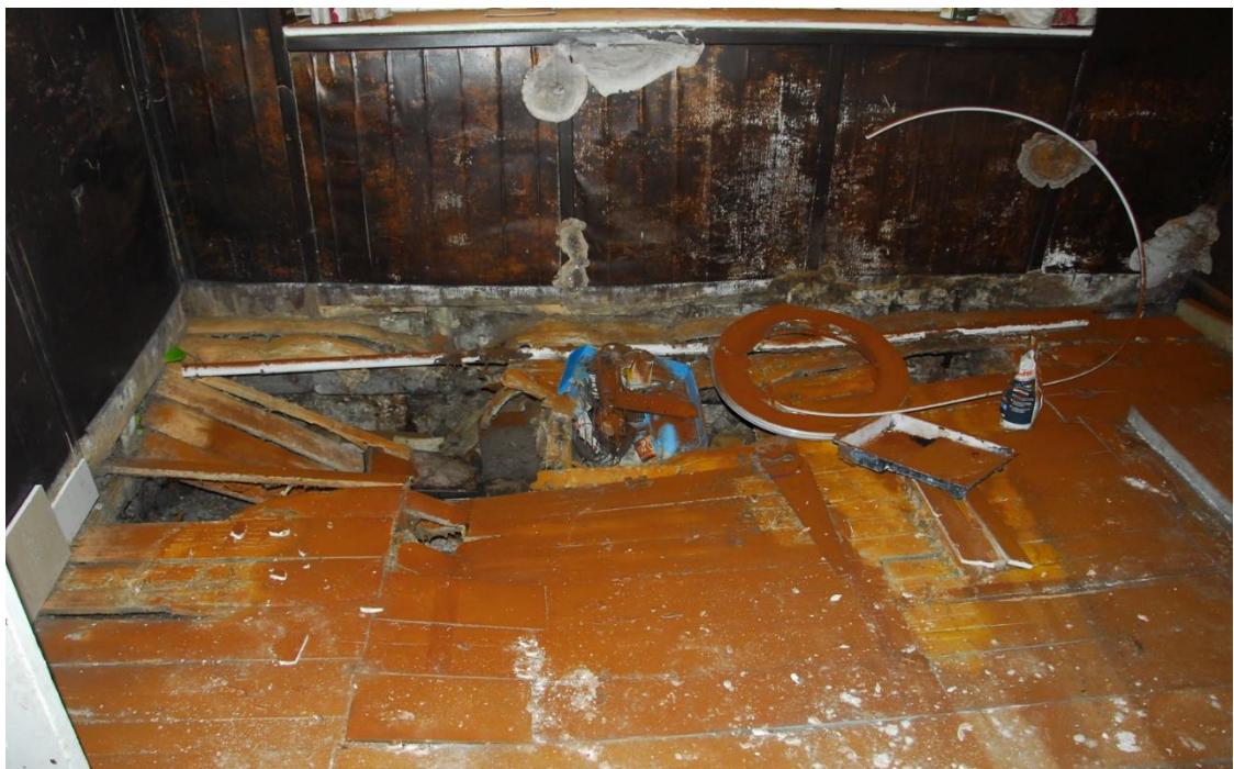
Figure 53 G7 panelling with fungal activity.
