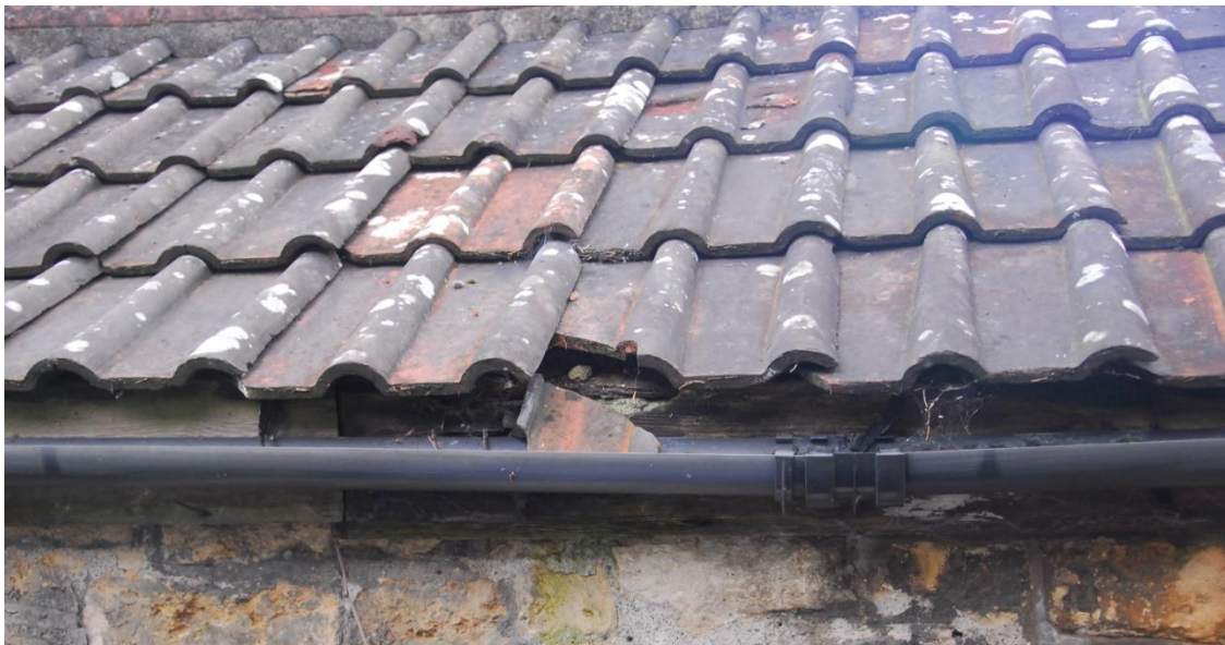
Figure 19 RS 11 Dislodged tiles most likely associated with top plate or rafter end failure
