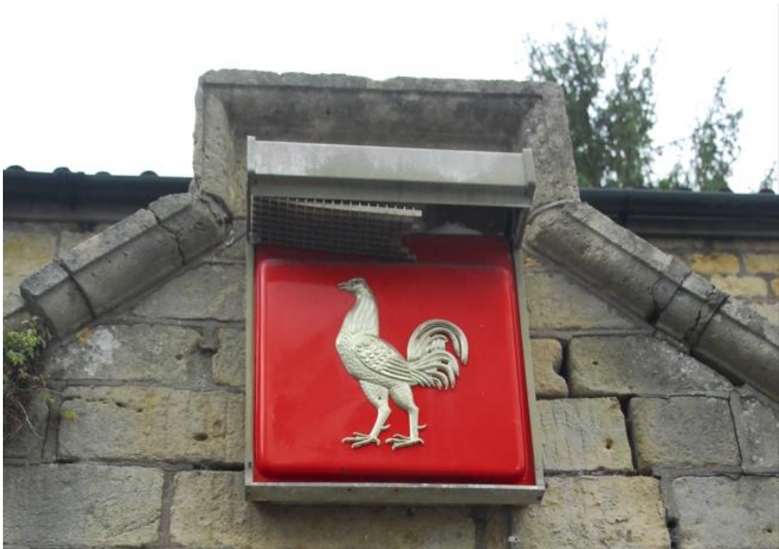
Figure 22 Awkward jointing to merlon and open joints.
