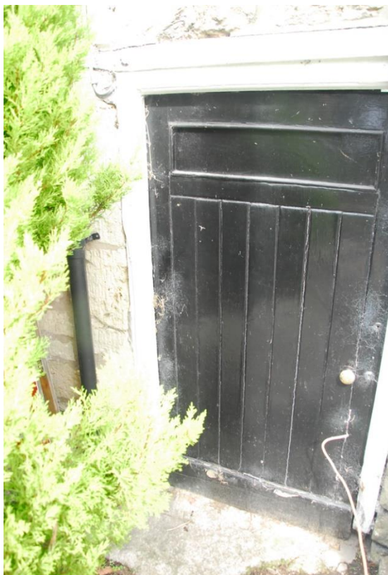
Figure 28 DG3 boarded door
