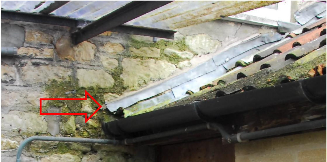
Figure 17 RS 10 kitchen and ladies toilets abutment with main building. Failed flashings
