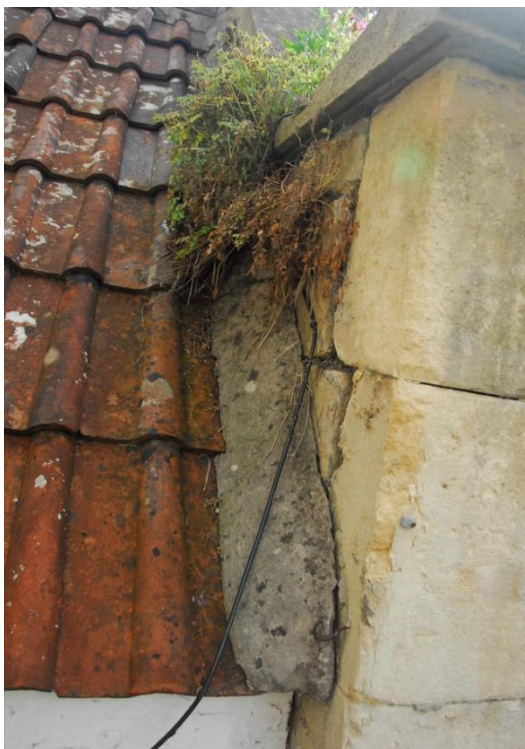
Figure 8 Porch abutment flaunching
