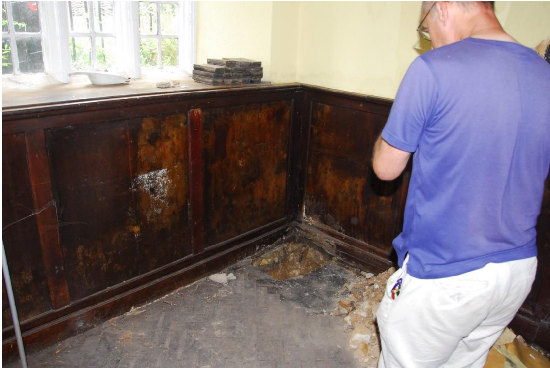
Figure 48 G1 Walls and panelling (saturated)
