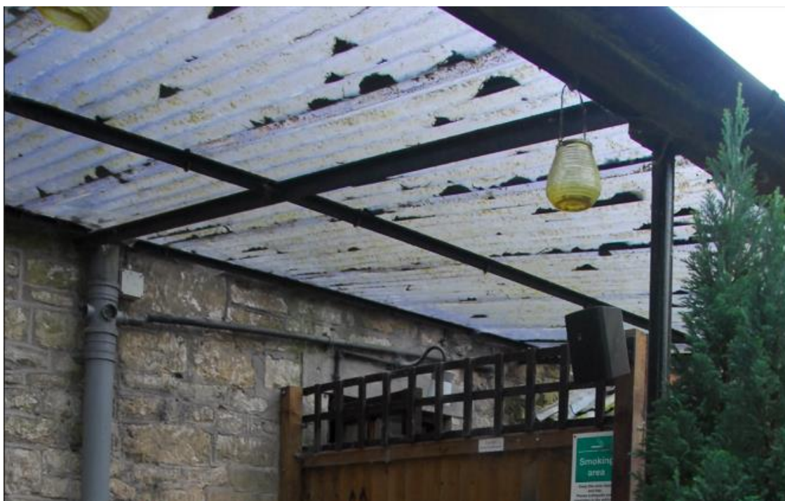
Figure 15 Inappropriate corrugated plastic roof which should be removed and is unlikely to be consented
