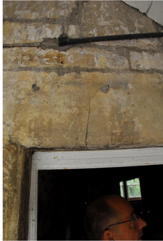
Figure 27 Fractured lintel over DG2
