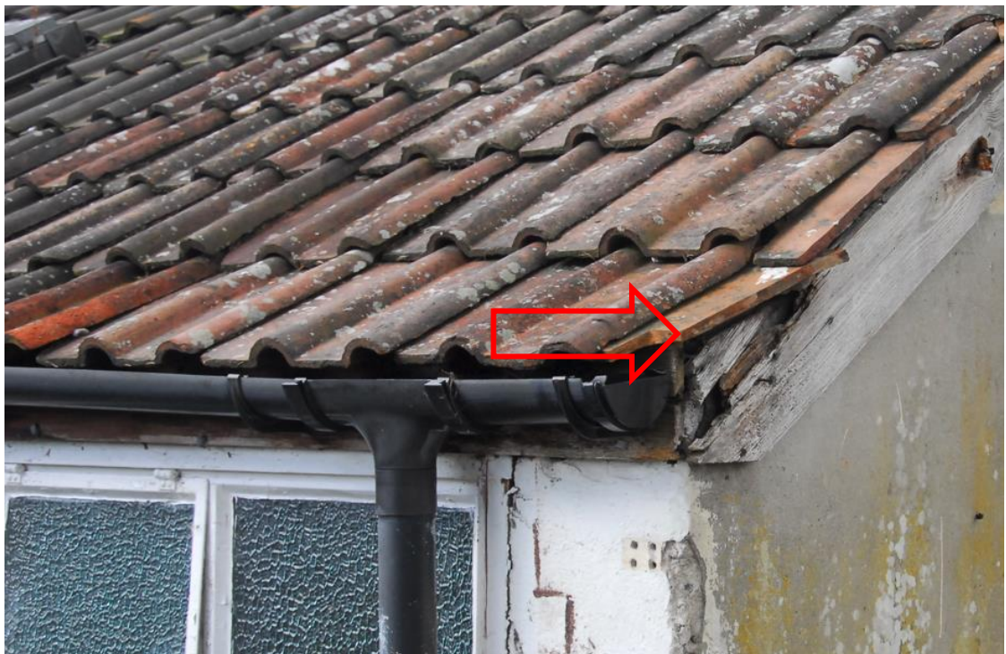
Figure 18 RS 10 kitchen and ladies toilets abutment with main building. Failed verge board
