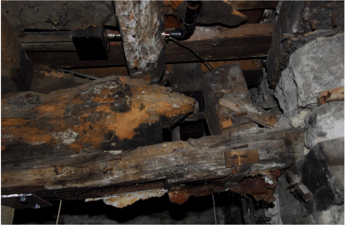
Figure 45 G3 failed western floor carrier
