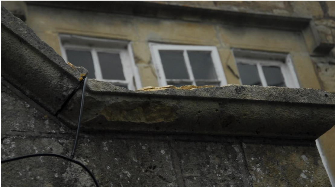
Figure 23 Failed horizontal coping
