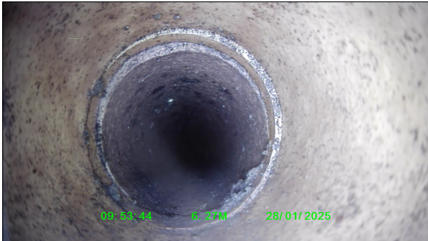
Photo: 4_4_53_A.jpg 6.3m, Fracture, circumferential at joint, from 12 to 12 o'clock
