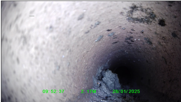
Photo: 4_4_48_A.jpg 2.1m, Settled deposits, fine, 15% cross-sectional area loss, Start
