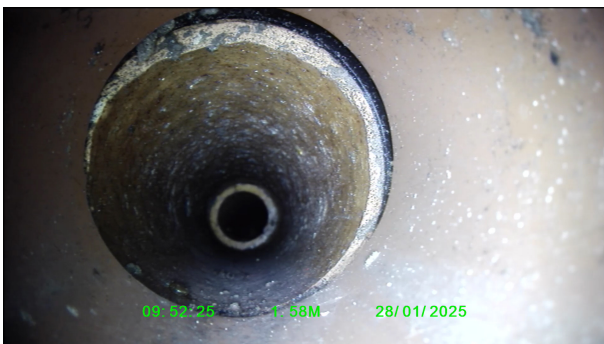
Photo: 4_4_45_A.jpg 1.7m, Open joint, medium Remarks: joint pulled
