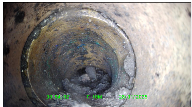
Photo: 4_4_75_A.jpg 7.3m, Survey abandoned Remarks: unable to pass beyond this point
