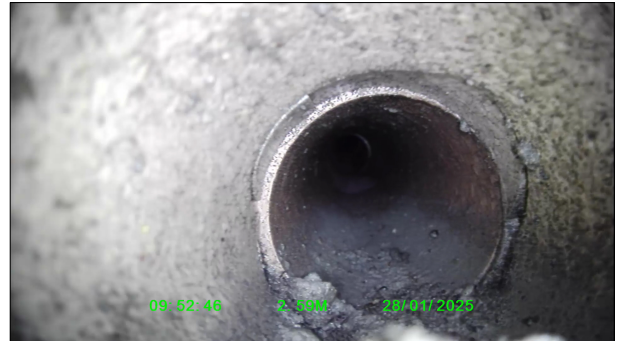
Photo: 4_4_49_A.jpg 2.7m, Fracture, circumferential at joint, from 9 to 4 o'clock
