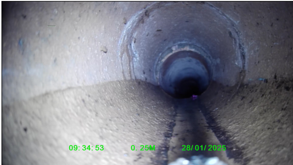
Photo: 3_3_27_A.jpg 0.4m, Fracture, circumferential, from 12 to 12 o'clock
