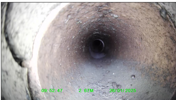
Photo: 4_4_50_A.jpg 2.7m, Line deviates up Remarks: joint pulled
