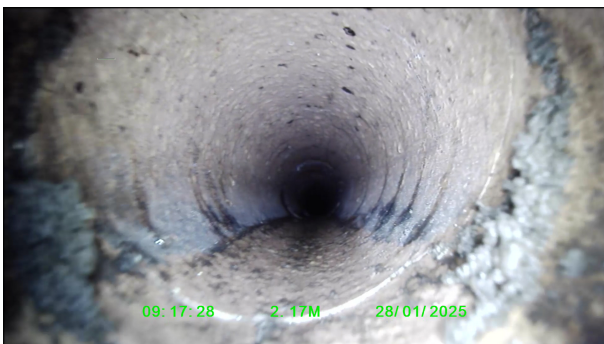
Photo: 1_1_10_A.jpg 2.2m, Fracture, circumferential at joint, from 2 to 7 o'clock
