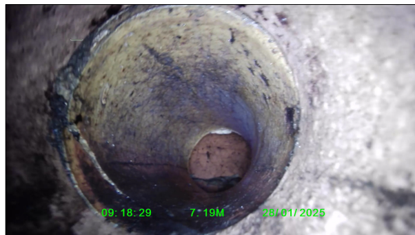
Photo: 1_1_19_A.jpg 7.2m, Fracture, circumferential at joint, from 6 to 9 o'clock
