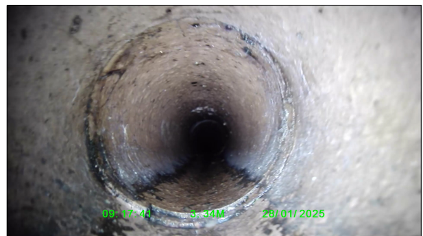
Photo: 1_1_11_A.jpg 3.4m, Fracture, circumferential at joint, from 3 to 9 o'clock
