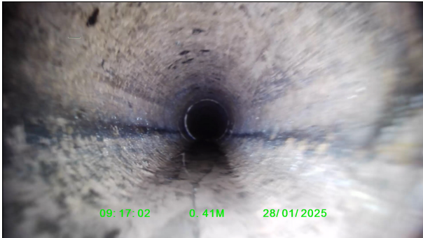
Photo: 1_1_7_A.jpg 0.5m, Fracture, longitudinal at joint, at 6 o'clock, Start
