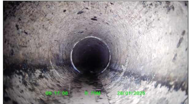
Photo: 1_1_8_A.jpg 0.8m, Crack, circumferential, from 4 to 10 o'clock
