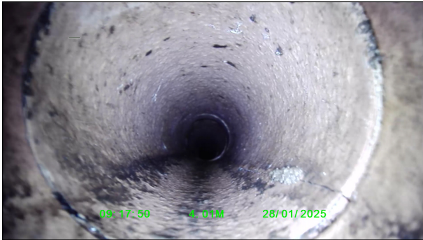
Photo: 1_1_12_A.jpg 4m, Fracture, longitudinal at joint, at 4 o'clock, Start
