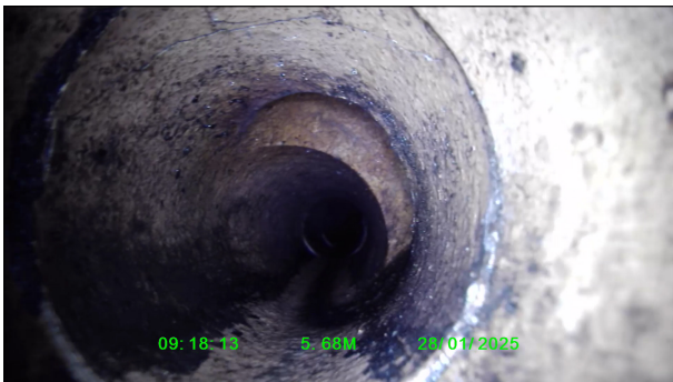
Photo: 1_1_15_A.jpg 5.7m, Crack, circumferential at joint, from 10 to 2 o'clock
