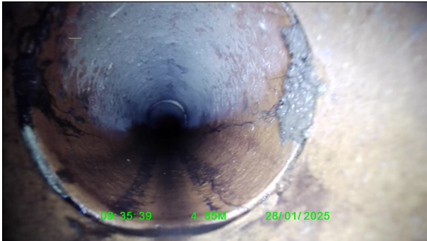
Photo: 3_3_31_A.jpg 4.9m, Roots, fine at joint
