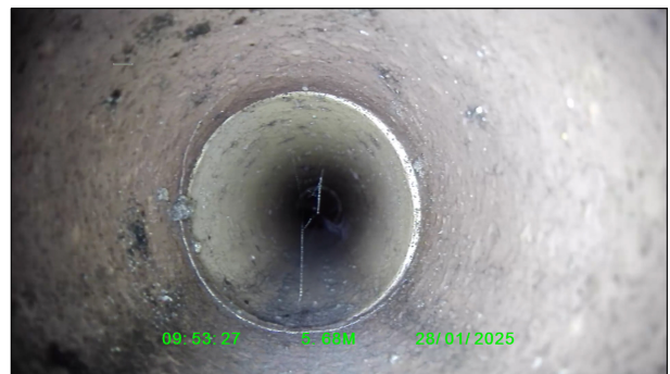
Photo: 4_4_52_A.jpg 5.8m, Crack, circumferential at joint, from 4 to 11 o'clock
