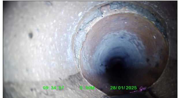
Photo: 3_3_28_A.jpg 0.6m, Joint displaced, medium Remarks: with flow
