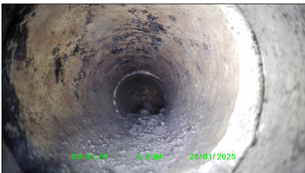
Photo: 4_4_56_A.jpg 6.8m, Settled deposits, fine, 10% cross-sectional area loss, Start
