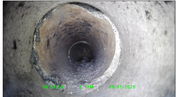
Photo: 4_4_54_A.jpg 6.8m, Broken pipe at joint, from 12 to 2 o'clock
