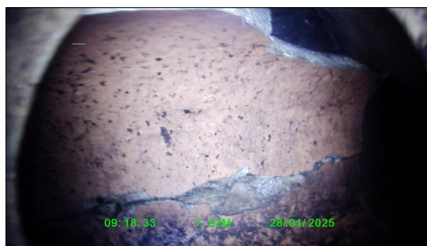
Photo: 1_1_21_A.jpg 7.6m, Attached deposits, fouling, from 12 to 12 o'clock, 5% cross-sectional area loss, End Remarks: vision obscured
