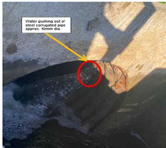
Figure 7- Defect at inlet (pipe close up).
