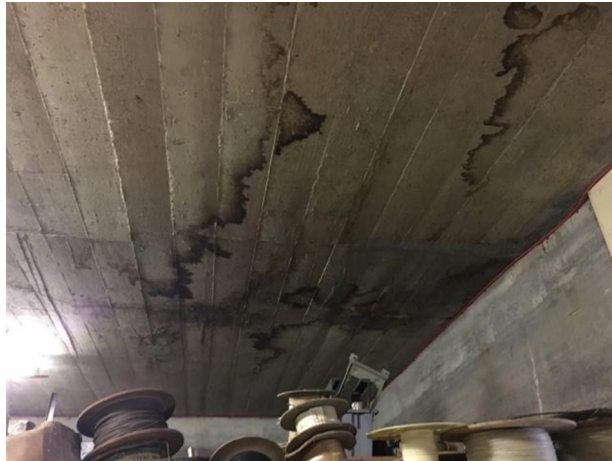
Image of the underside of the deck shows a number of leaks
