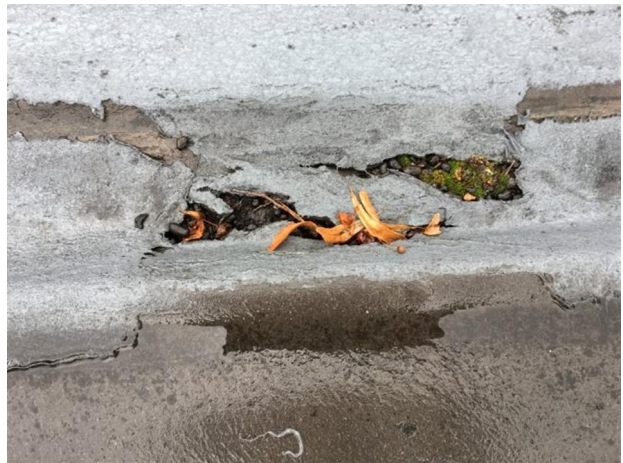
Further evidence of damaged waterproofing to the perimeter detail
