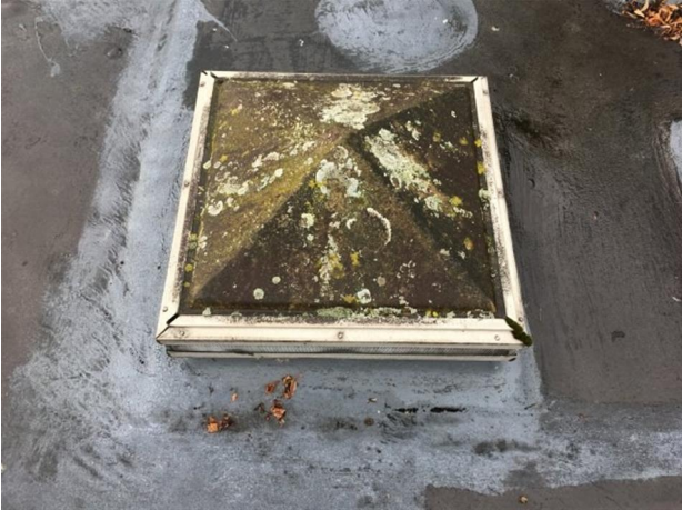
The existing rooflights are aged and should be replaced or removed all together
