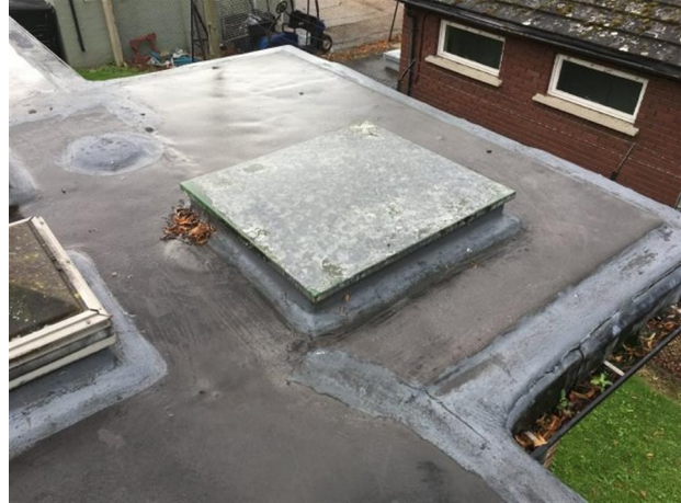
Access hatch covers a manhole cover and therefore must be retained. The kerbs must be dressed in new waterproofing.
