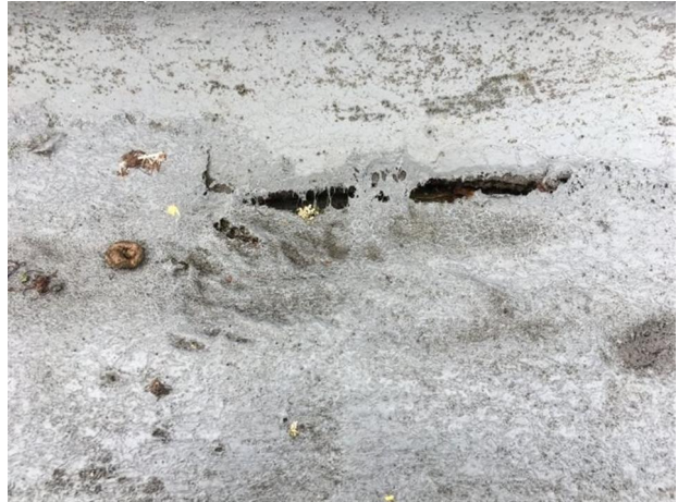
Evidence of splits in the asphalt at the upstand to rooflight
