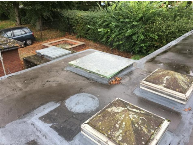
Extensive liquid repairs show an evidence of water ingress
