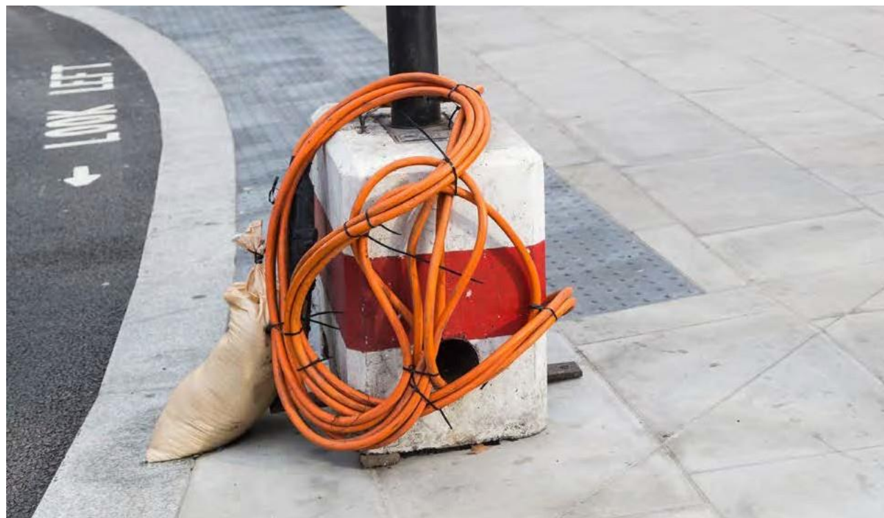
PTS cables should not be easily accessible
