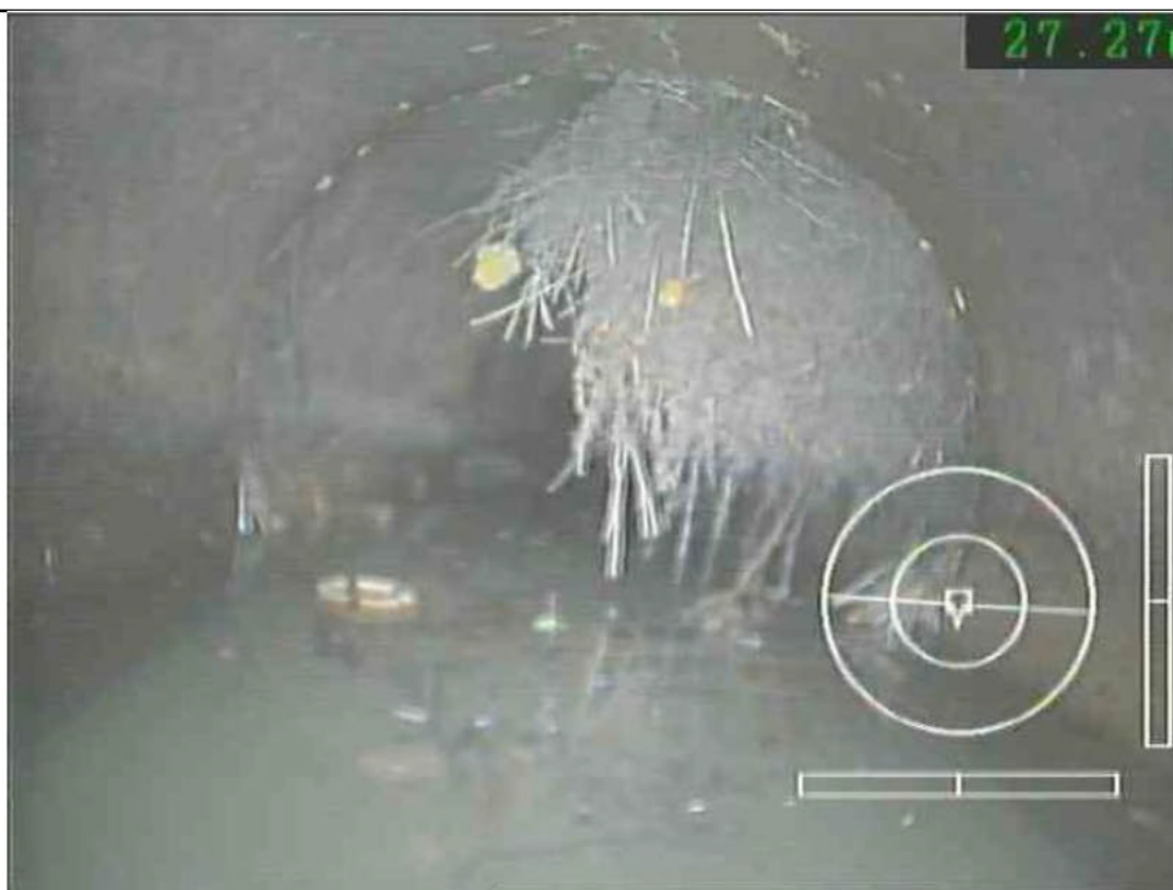
Figure 4 - CCTV photo of 45% blockage.
