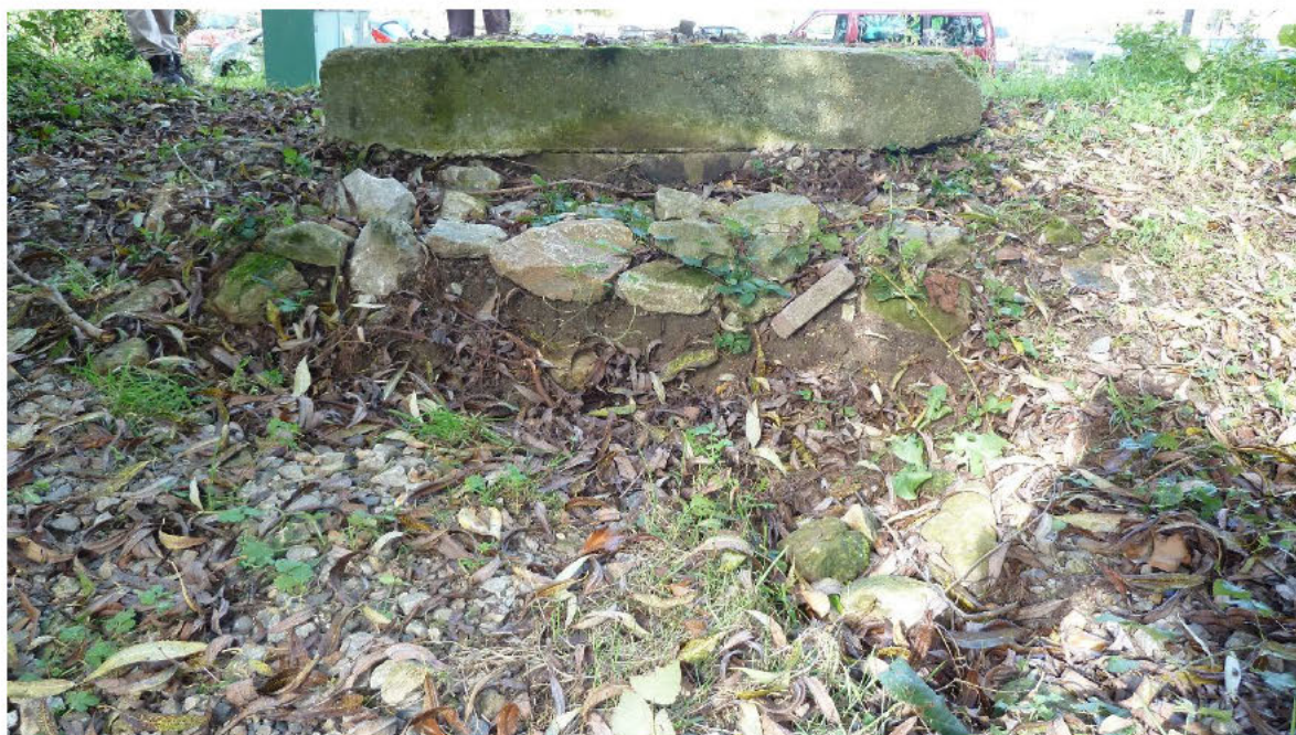
Figure 3 - Erosion on exposed face of embankment at MH1.
