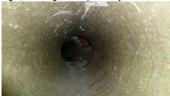
Figure 6 – Inlet to MH2
