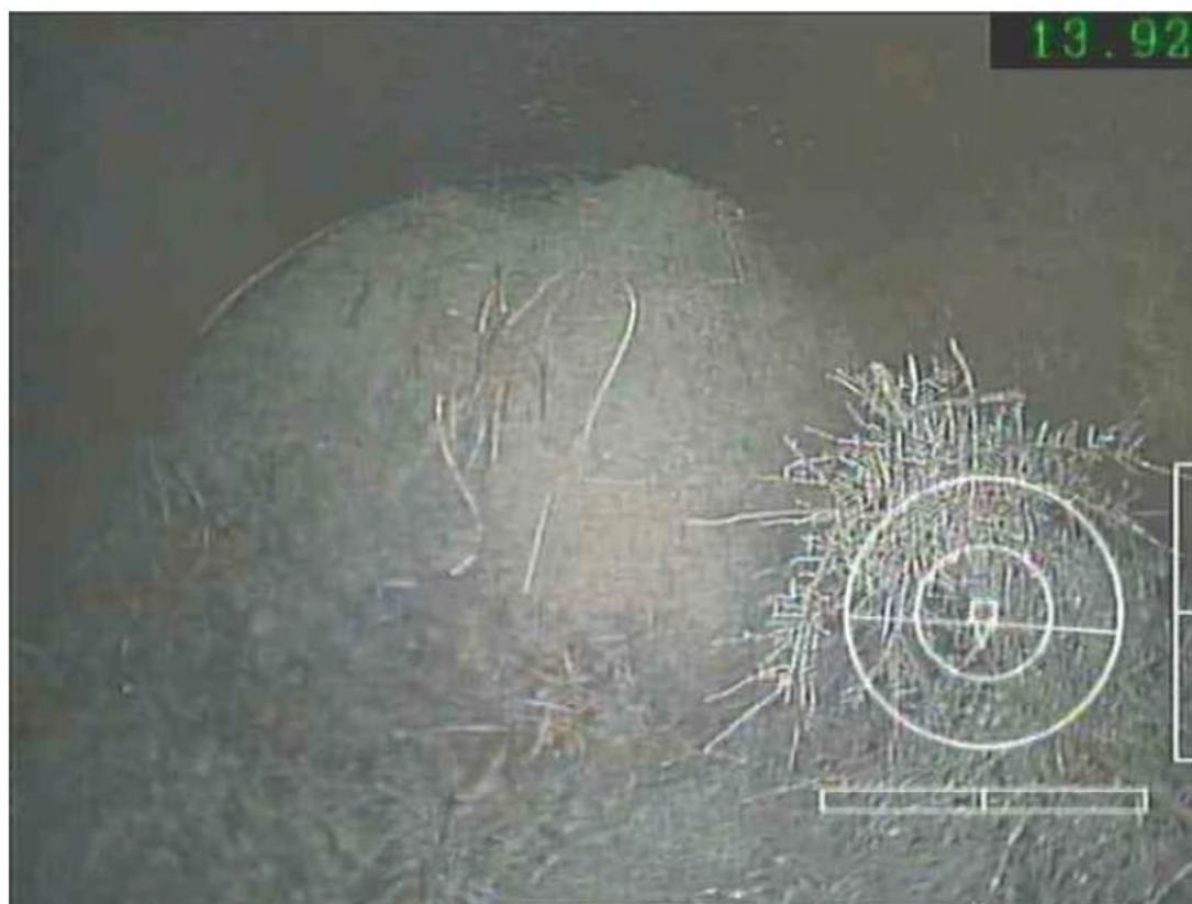
Figure 5 - CCTV Photo of 100% blockage.
