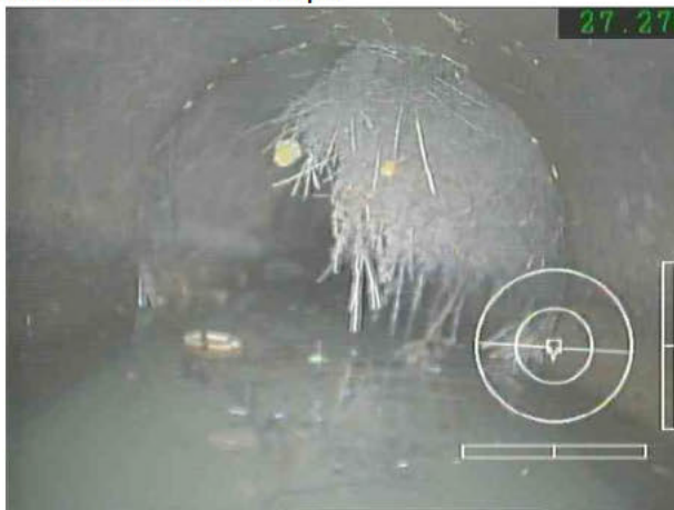
Figure 4 [repeated] - CCTV photo of 45% blockage
