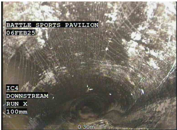
1, 00:00:04, 0.30 m Deformed sewer or drain, 10%, start
