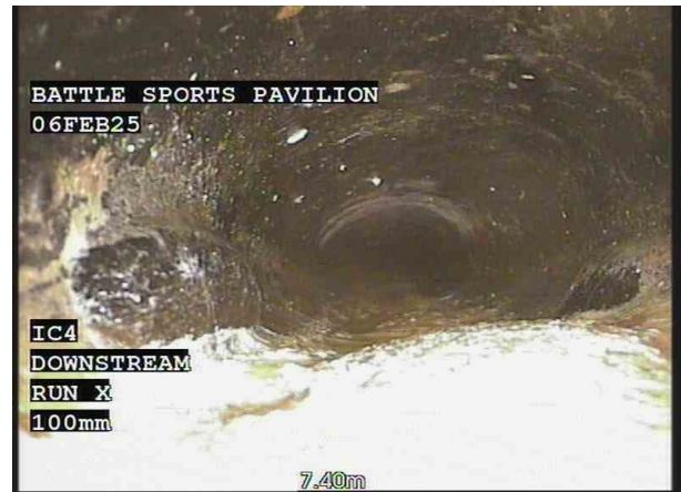
2, 00:00:56, 7.40 m Deformed sewer or drain, 20%, start
