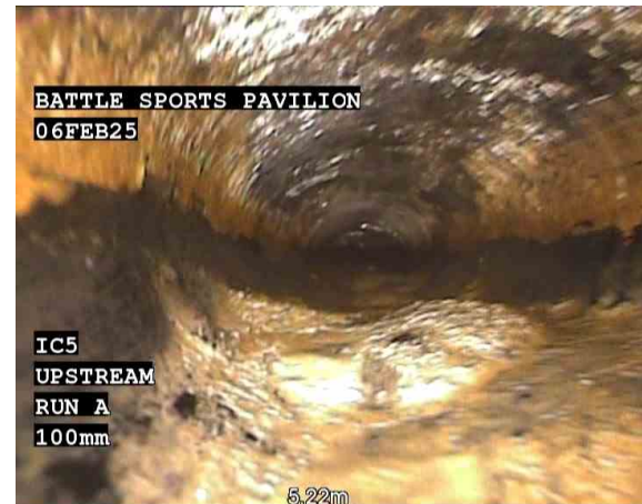
2, 00:00:27, 5.22 m Deformed sewer or drain, 20%, start
