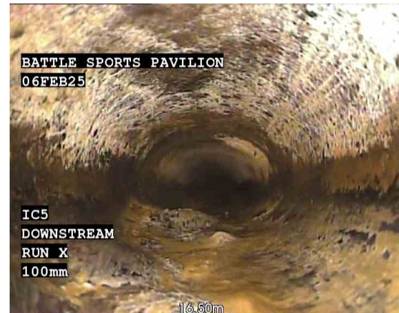
2, 00:00:41, 16.50 m Deformed sewer or drain, 10%, start
