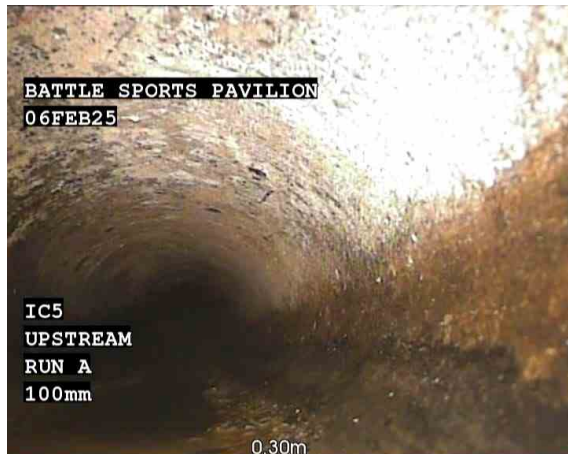
1, 00:00:00, 0.30 m Deformed sewer or drain, 10%, start
