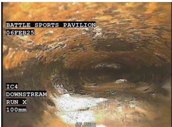
3, 00:04:06, 67.83 m Deformed sewer or drain, 40%, start
