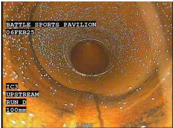
1, 00:00:27, 1.97 m Crack, circumferential from 03 o'clock to 06 o'clock
