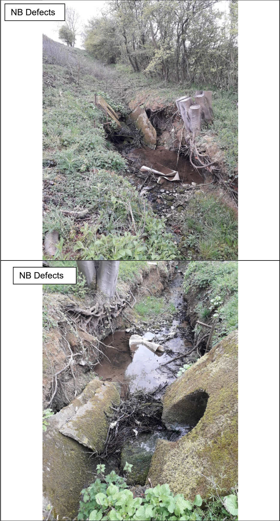
Figure 6-12: Photographs of major defects (Ratcliffe)
