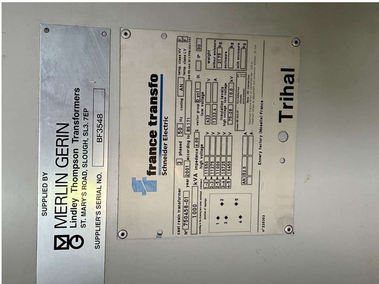
CBRM Transformer Name Plate
