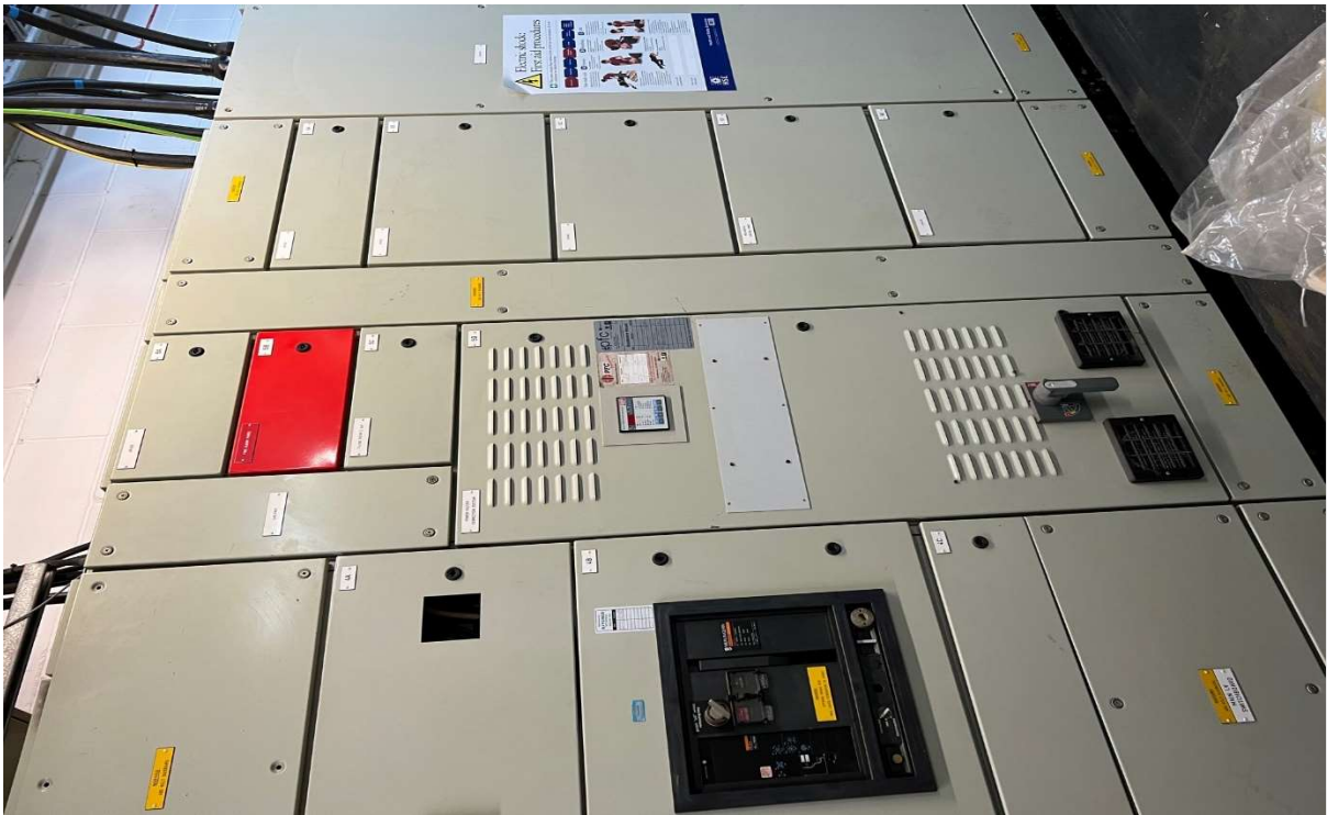
Existing LV Switchboard
