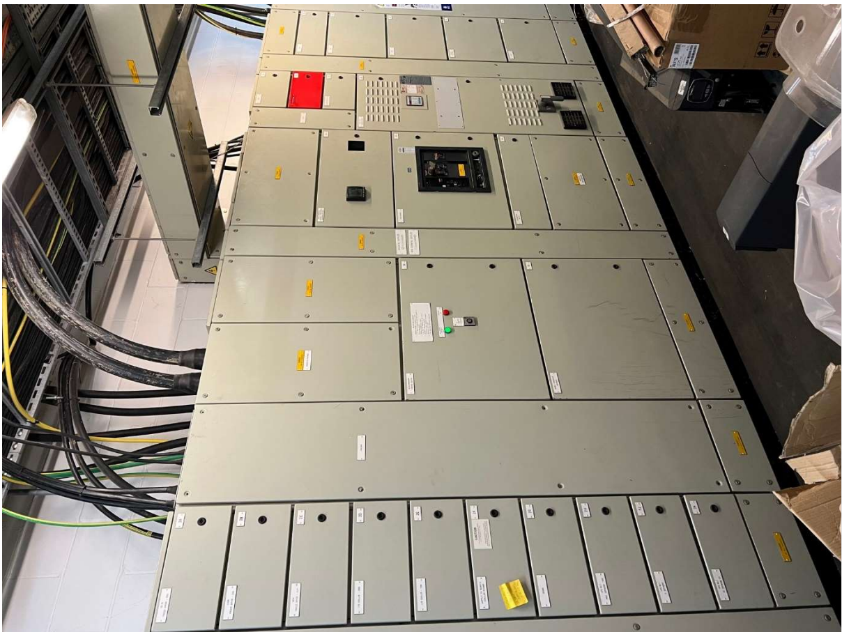
Another view of LV Switchboard
