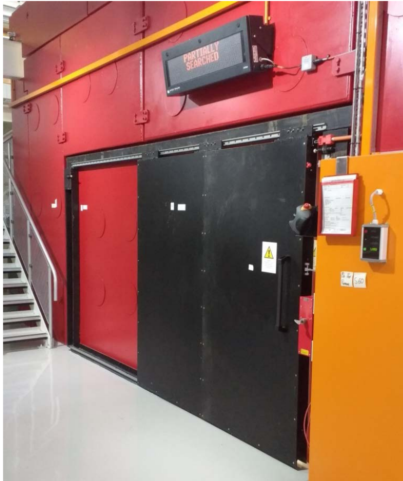
Figure 1 – Existing IMAT manually operated shield door
