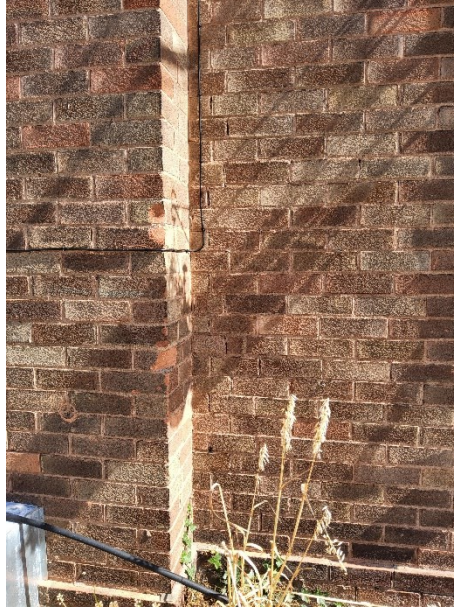
Figure 5 – Crack to brickwork next to chimney (side elevation)
