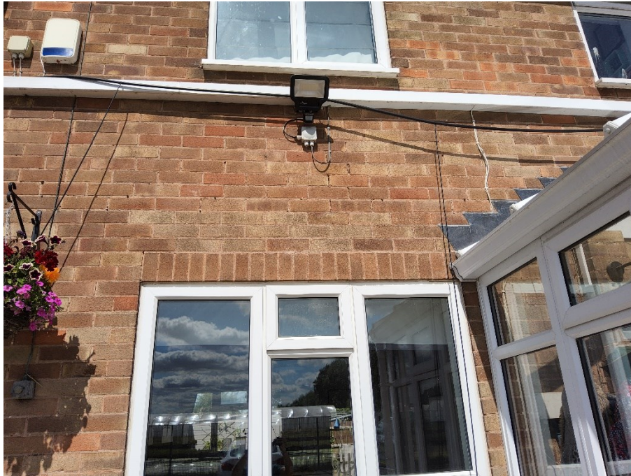
Figure 3 - Cracking above window (front elevation)
