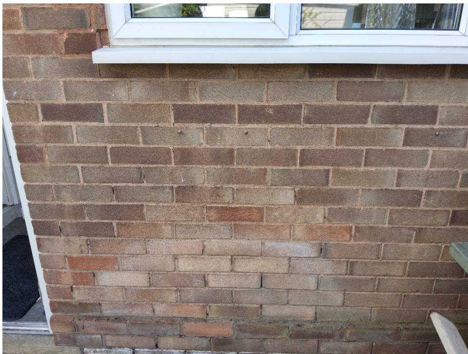
Figure 8 –Mortar loss below window (rear elevation)
