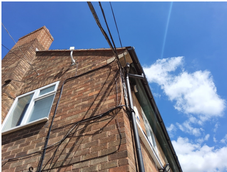
Figure 4 – Crack and displaced brick to top corner of building
