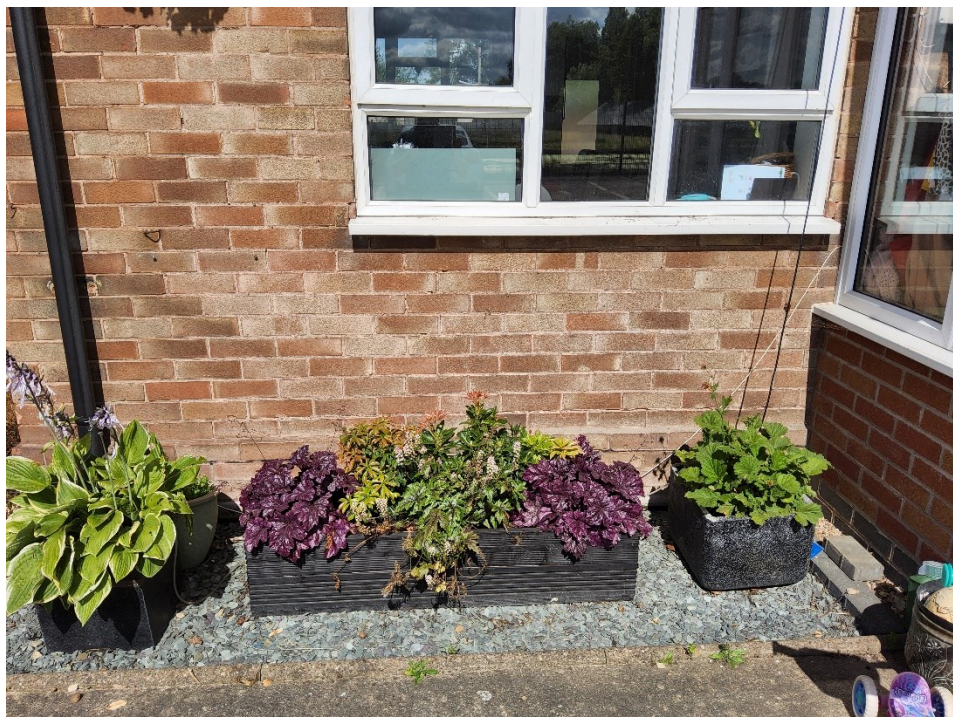
Figure 2 – Stepped crack below window (front elevation)
