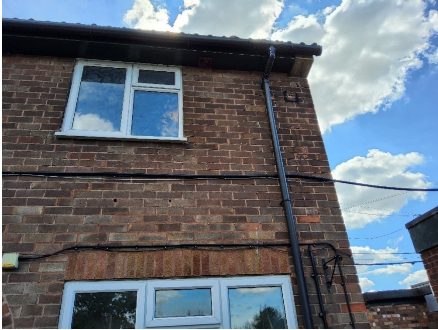
Figure 9 – Mortar loss and minor cracking
