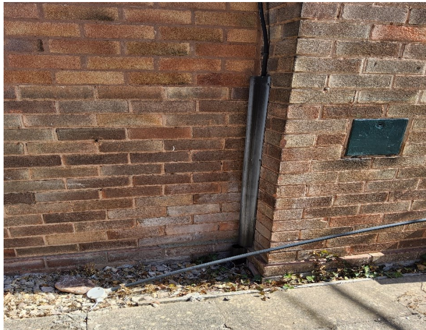
Figure 6 – Minor crack to lower section of wall next to chimney (side elevation).
