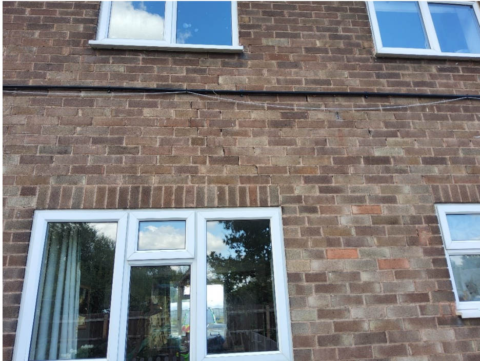
Figure 11 – Stepped cracking over window (rear elevation)
