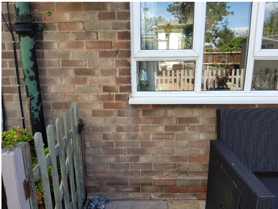
Figure 12 – Further cracks probably due to drainage leakage.
