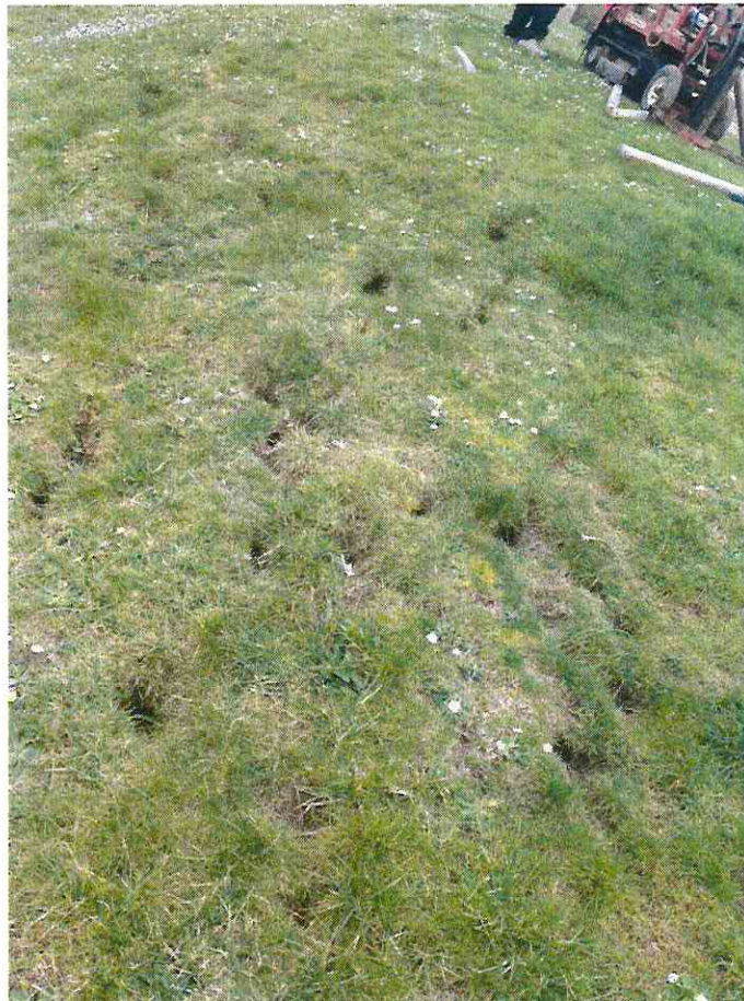
Tension cracks within crest of slope above southern end of site, adjacent to WS9.
