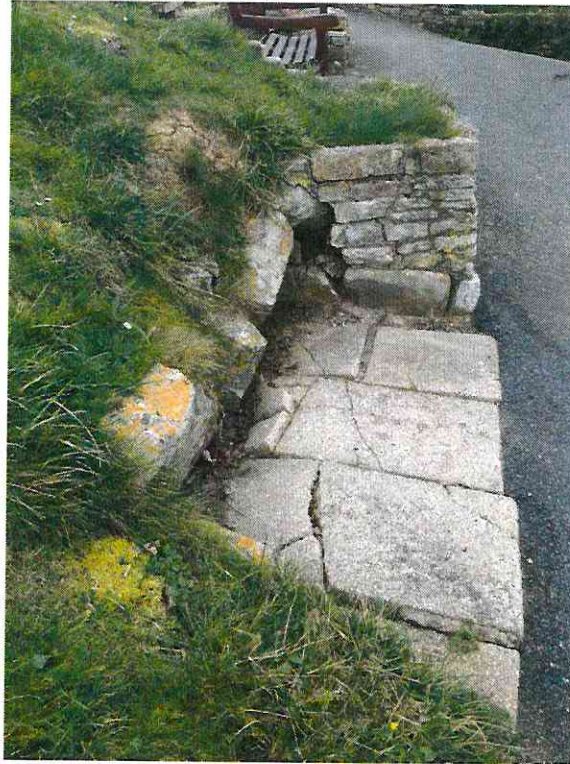
Slumping wall and cracked paving slabs.
