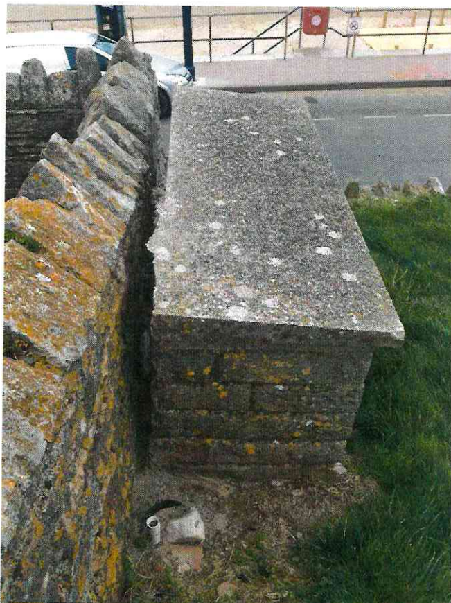
Slumped electrical box. Formerly attached to stone wall to the left.
