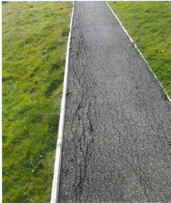
View of pathway in middle part of site showing signs of slippage.
