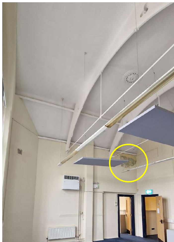
Figure 8: Photograph in Area R5 showing evidence of water ingress
