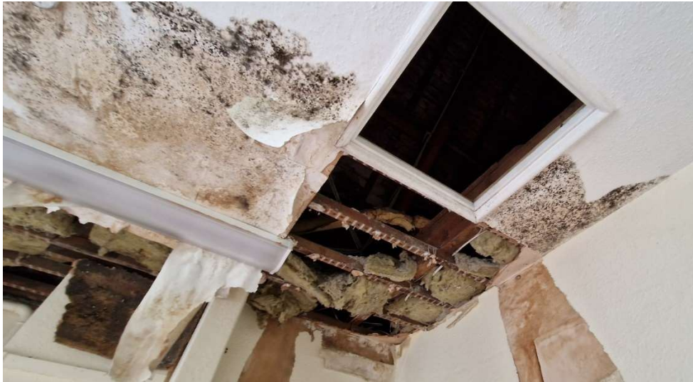
Figure 31: Photograph of collapsed ceiling around access hatch
