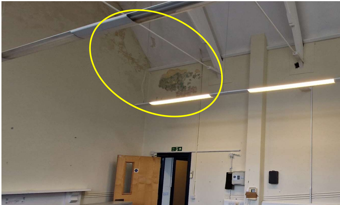
Figure 9: Photograph in Area R6 showing evidence of water ingress
