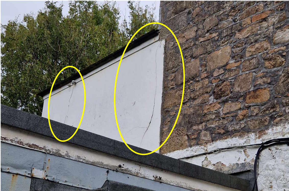
Figure 38: Photograph showing vertical crack on the west elevation of White House
