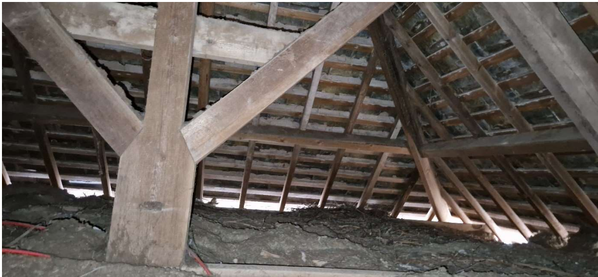
Figure 6: Photograph within roof space R3 showing King Post truss and evidence of animal ingress
