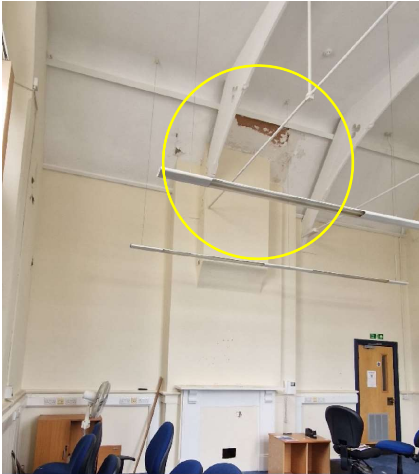
Figure 12: Photograph of Area R9 showing evidence of water ingress around chimney
