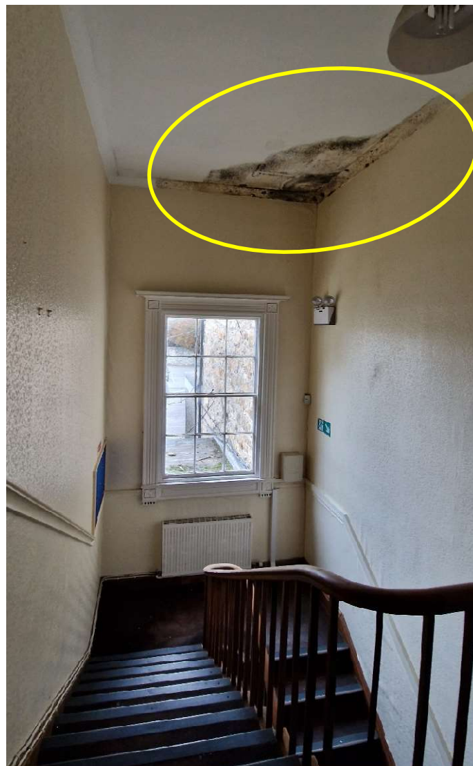
Figure 27: Photograph showing water ingress over main stair half landing
