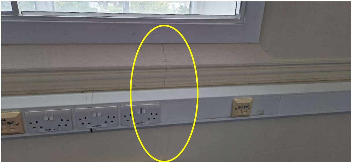
Figure 15: Photograph of vertical cracking beneath first floor window openings
