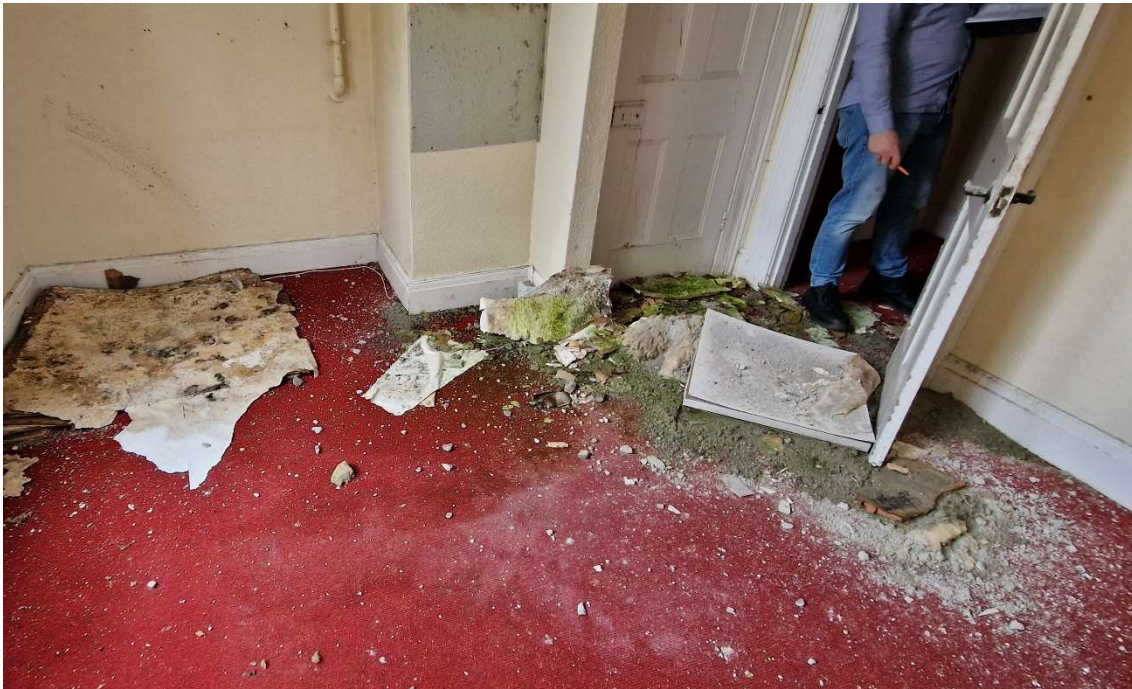
Figure 29: Photograph showing remnants of collapsed ceiling at first floor
