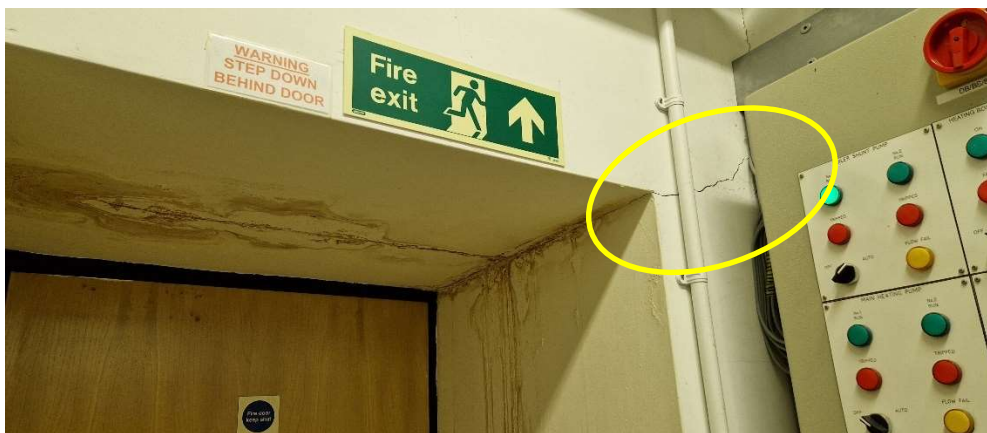
Figure 20: Photograph showing cracking around the plant room door opening
