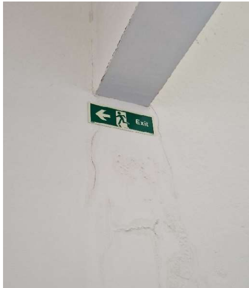
Figure 17: Photograph showing cracking at first floor steel beam bearing
