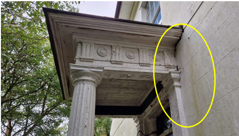
Figure 35: Photograph showing porch over main entrance to White House. Minor cracking/separation highlighted at interface with wall
