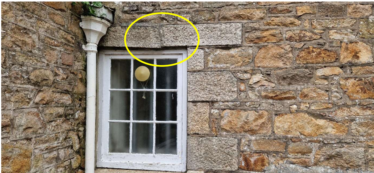
Figure 22: Photograph showing lintel failure over ground floor window opening
