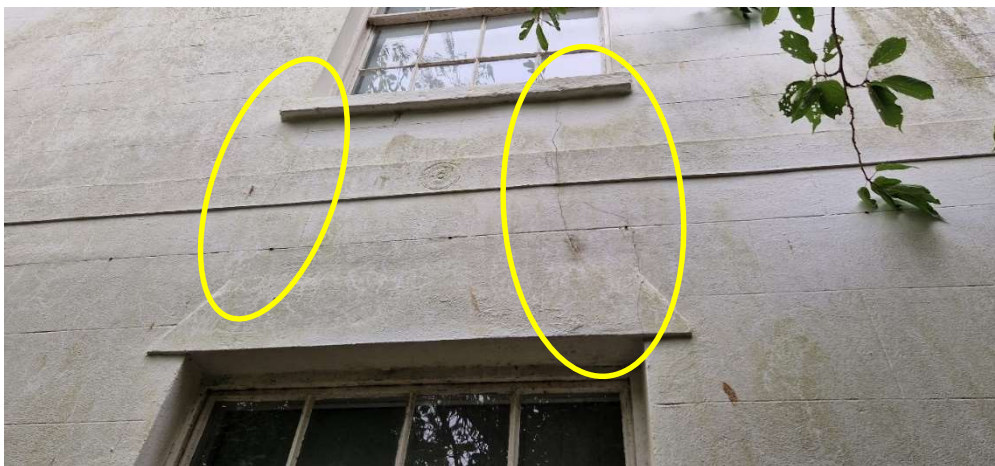
Figure 36: Photograph showing vertical cracking between window openings on front elevation
