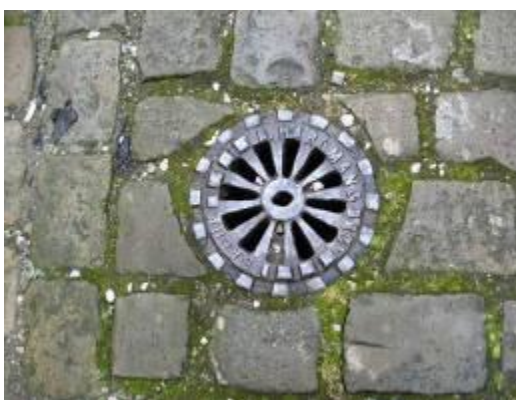
Drain cover in Bank Street
