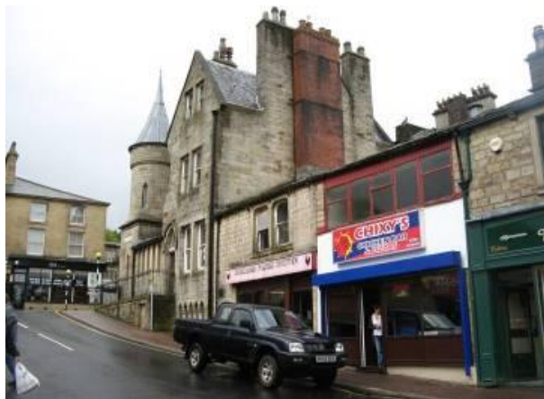
Poor quality shopfronts in Union Street
