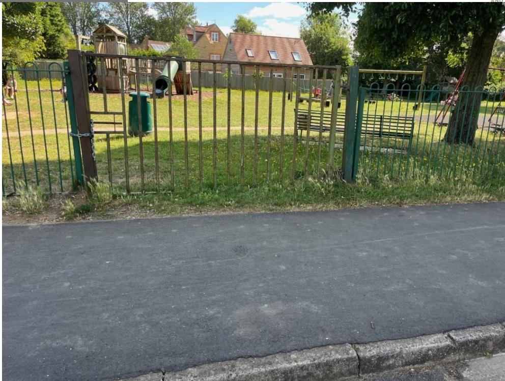
Photo Above: Maintenance Gate to access site – note there is no drop kerb.
