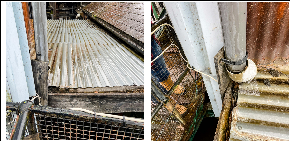
Screens: Roof over lamp room waiting area is very badly made. The sheets do not extend to the edge and the RWP from the upper roof soaks the gap
