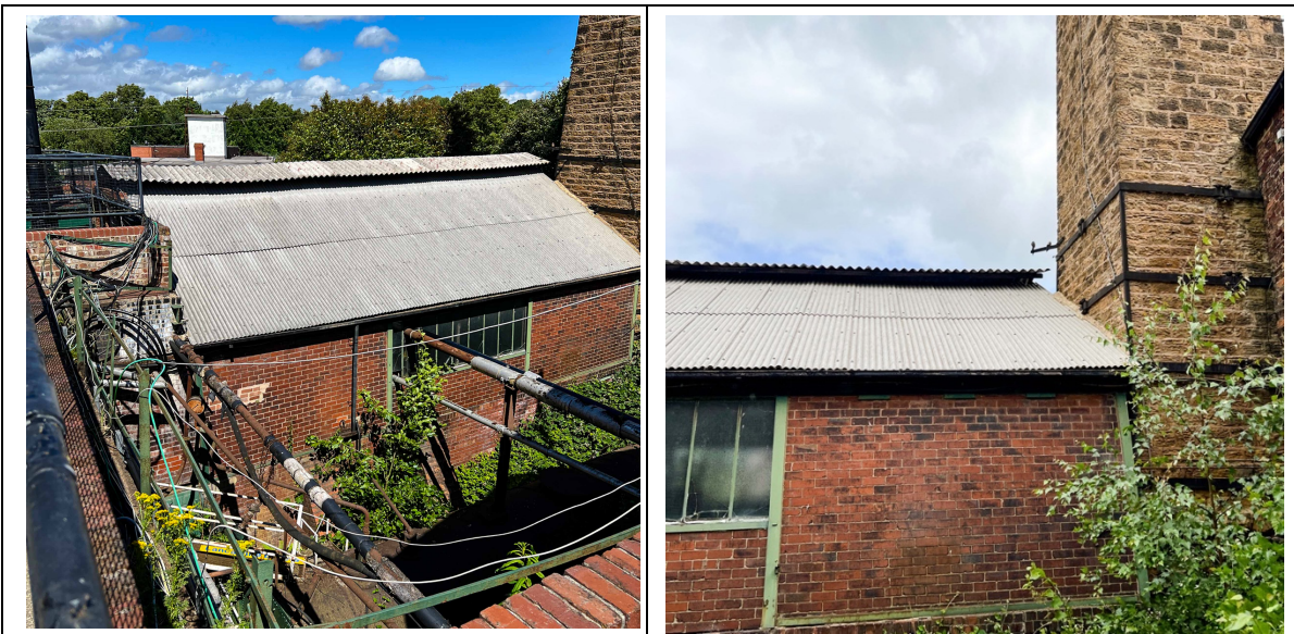
Lancashire boilers. Replace eaves gutters
