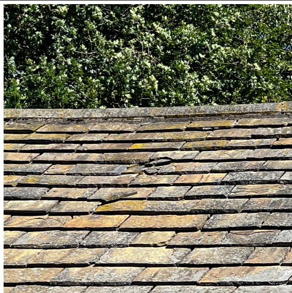
Roof: North side damaged roof slates
