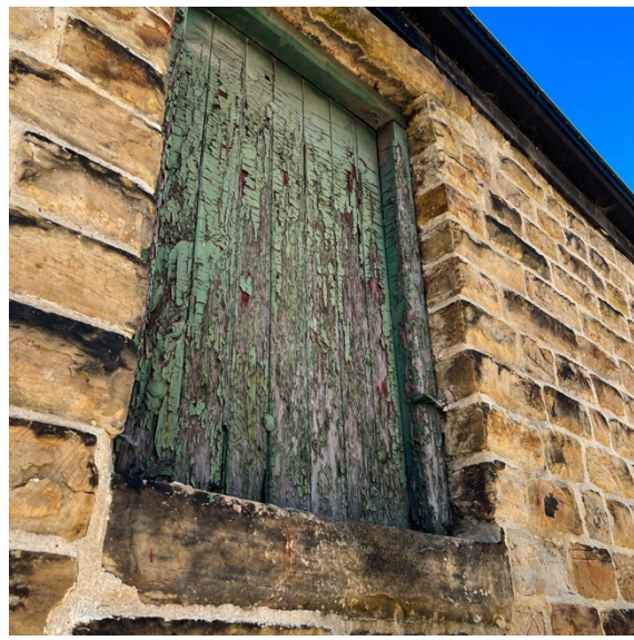
South. Door in poor order
