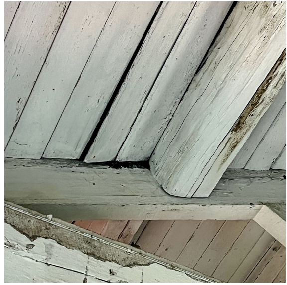
Interior: ceiling boards need refixing
