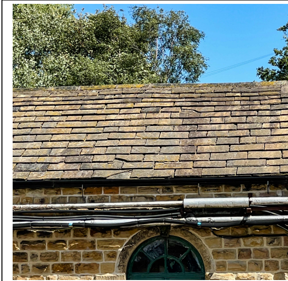
Roof: Cracked and broken slates to North side
