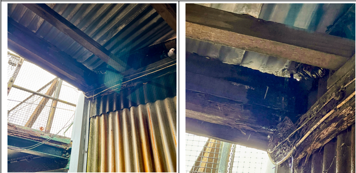
Screens: Underside view of above showing soaked and rotten timbers
