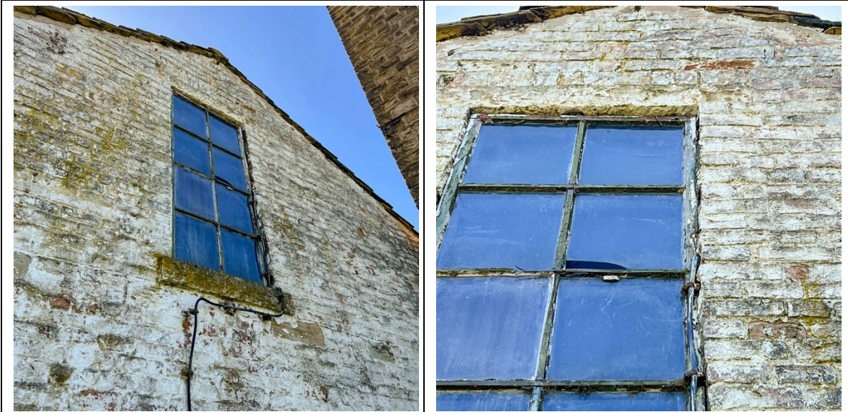
East. Window in poor order. Elevation needs limewashing
