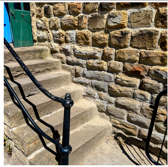
Elevations: North steps, mortar falling from joints and gathering on steps
