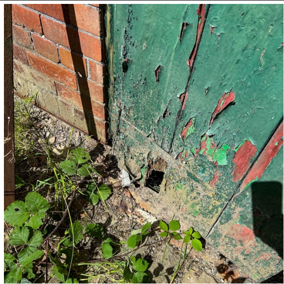
Lancashire boiler - Switch room door to replace
