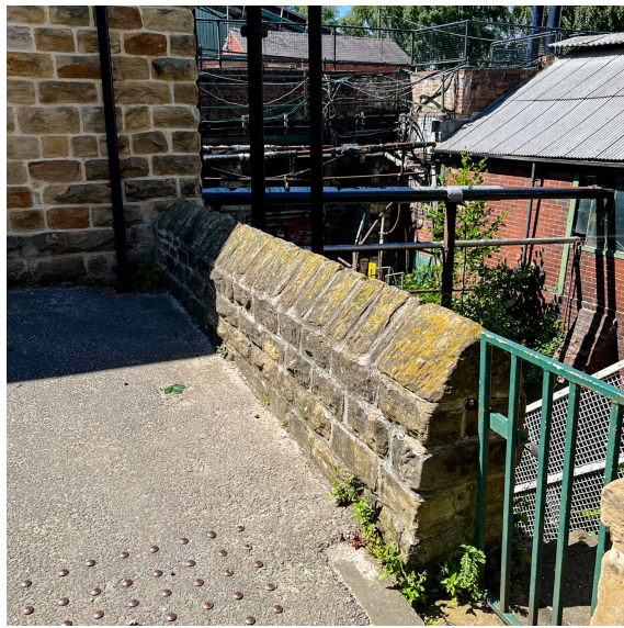
West elevation, Low wall could do to have a guard rail 1.1m high
