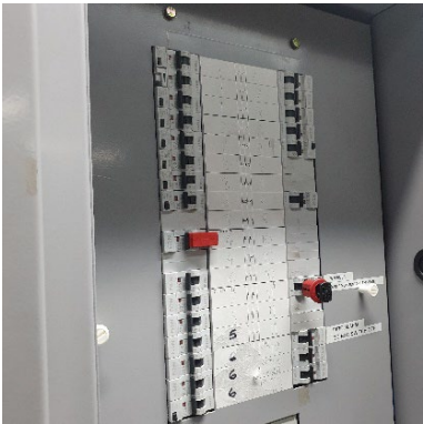
Fig 6- MCB with example push lock circuit breaker lockout device
