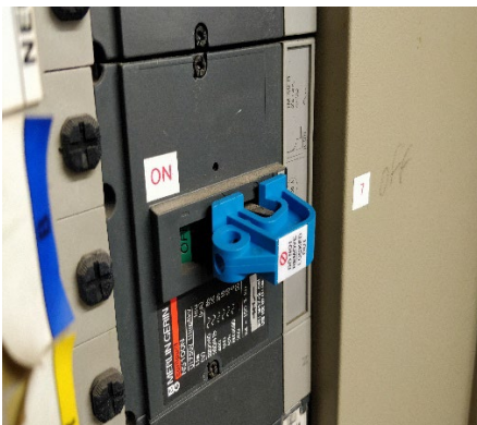
Fig 3- Universal circuit breaker lockout
